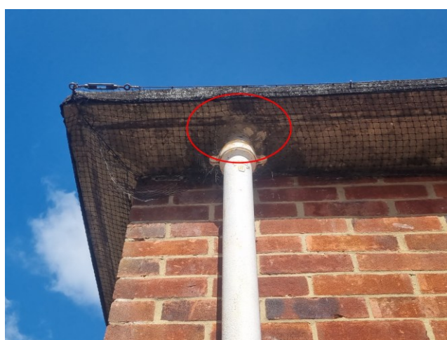
Photograph 11. Gaps in the netting around a down pipe.
