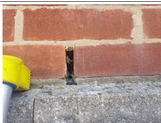
Photograph 6. Weep vent blocked with debris and cobwebs.
