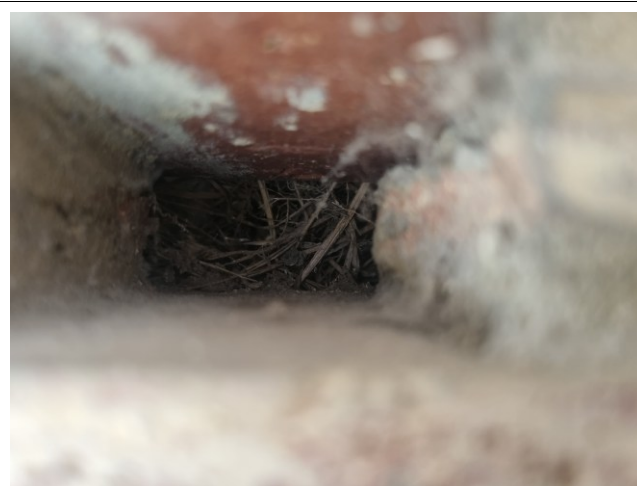
Photograph 10. Nesting material within the wall vent.
