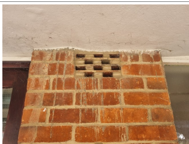
Photograph 3. Bespoke wall vent under the veranda.
