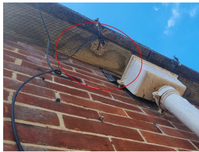
Photograph 12. Larger gap adjacent to a downpipe hopper.
