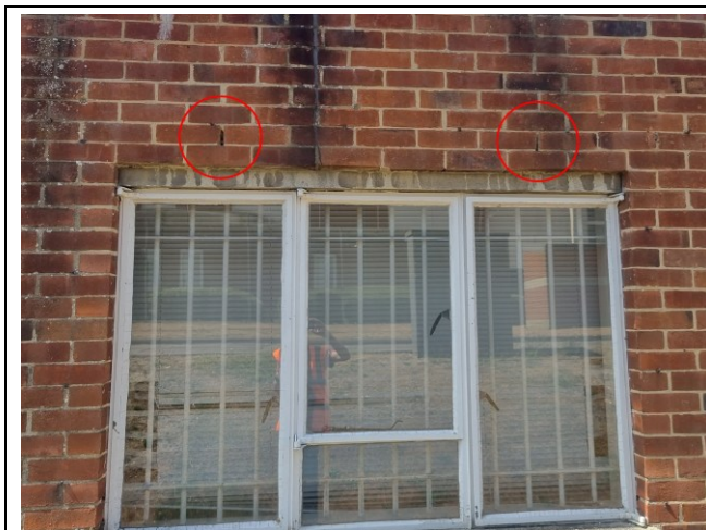
Photograph 5. Location of weep vents above a rear window.
