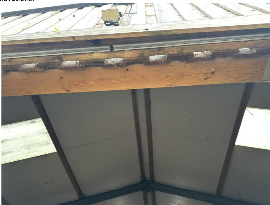
Photograph 7: Gaps along the top of the timber sliding door (Target Note 2), evident on both east and west elevations.
