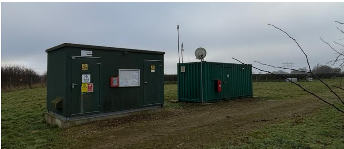
Photo 7: A Typical Item of Fixed Equipment
