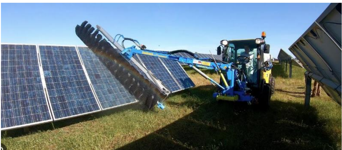
Cleaning of Solar Arrays
