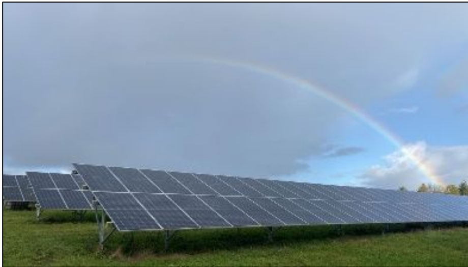
Photograph 6.1 - Typical view of a solar site ground coverage
