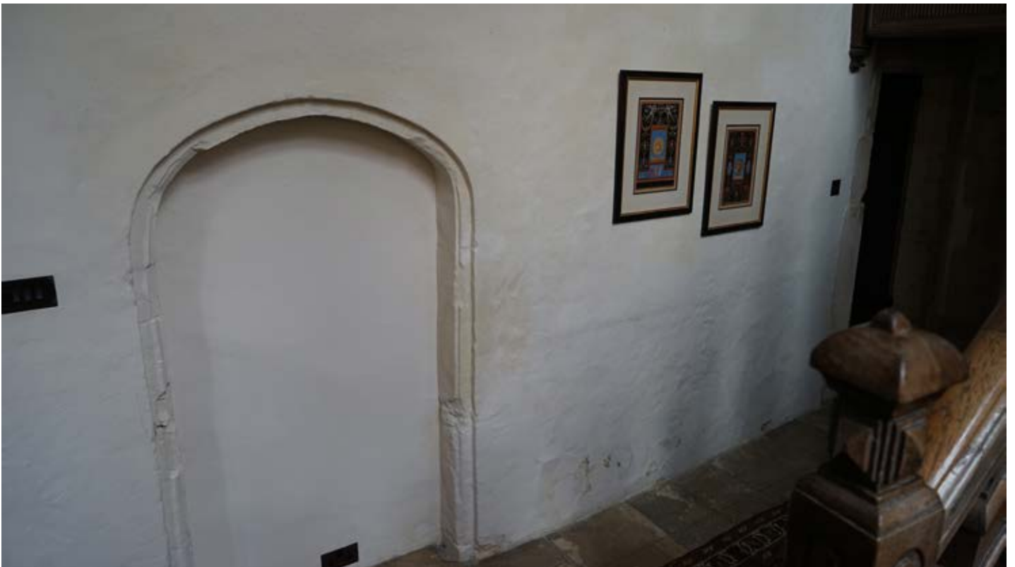
Blocked door opening from staircase passage.
