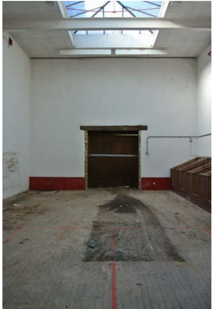
Squash court interior - Large opening formed in back wall.
