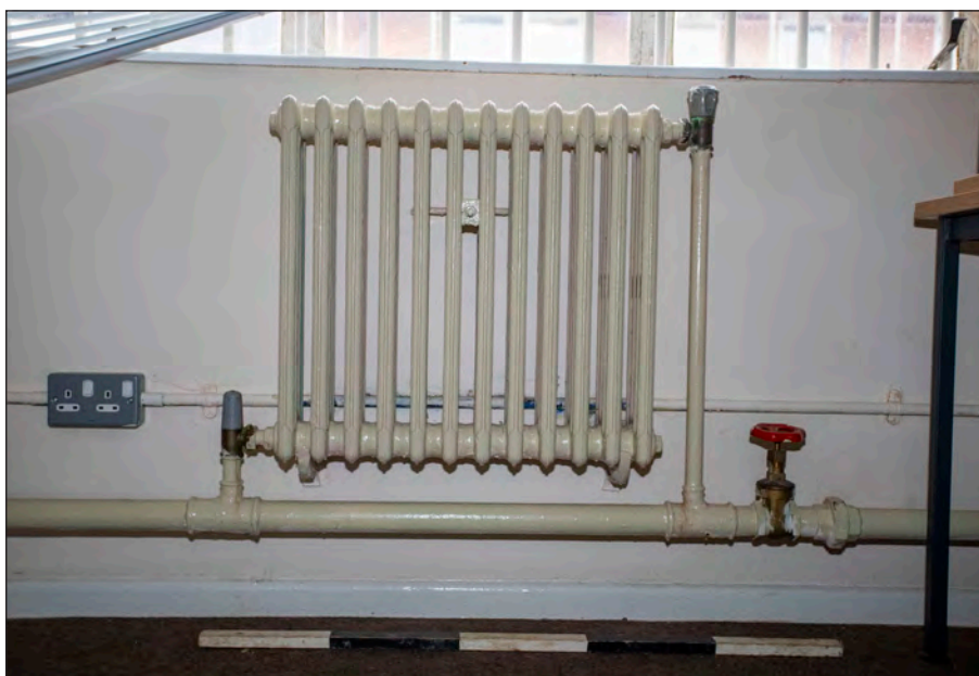
Photograph 30: Building JE 0 060 example of a cast-iron column radiator
