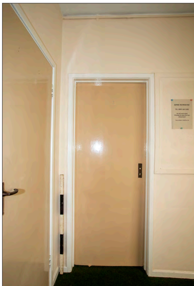
Photograph 33: Building JE 0 060 blocked door nailed shut between family room G65 and kitchen G66
