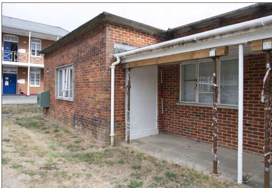
Photograph 11: Building JE 0 060 blocked entrance into the north-west end of the building
