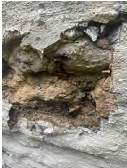
Area stripped of waterproof slurry to north elevation.
