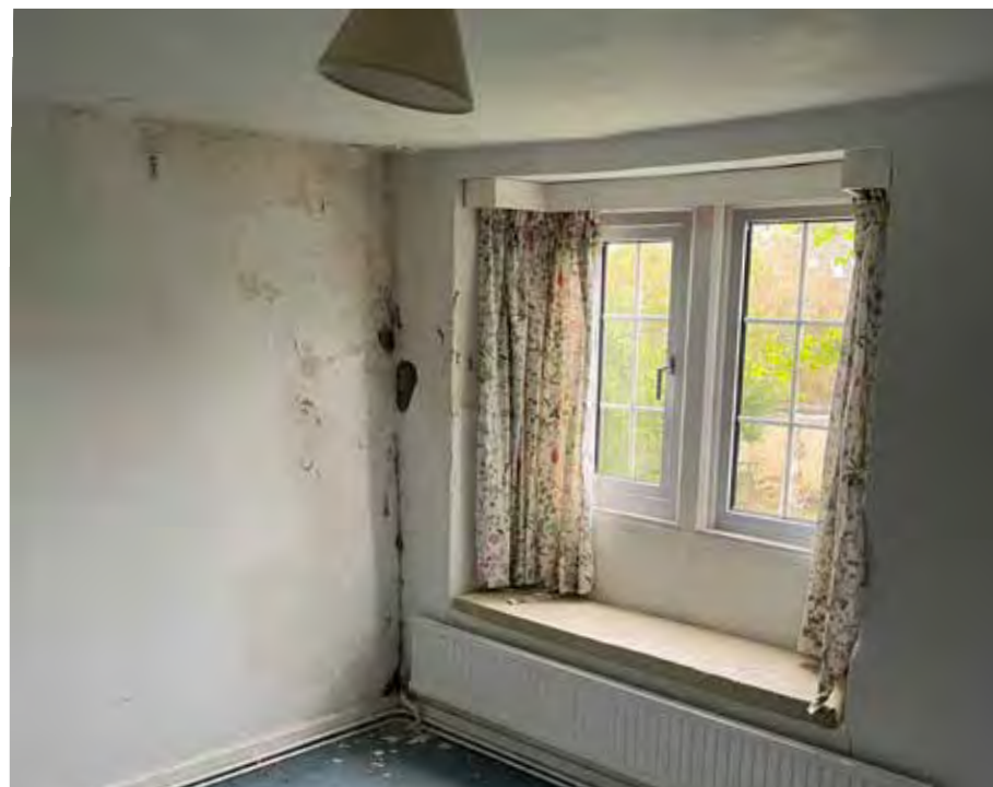
Internal view of first floor Bedroom One - Structural movement & damp | 2025
