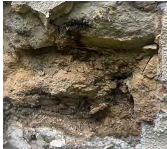
Detail showing powdered stonework beneath removed slurry to north elevation, with moisture content of 78%.
