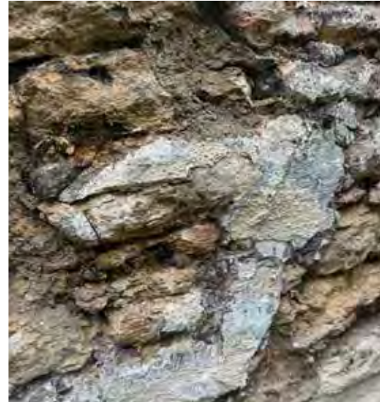
Area of removed cementitious render using hand tools to reveal powdered stonework and mortar beneath, with 70% moisture content.
