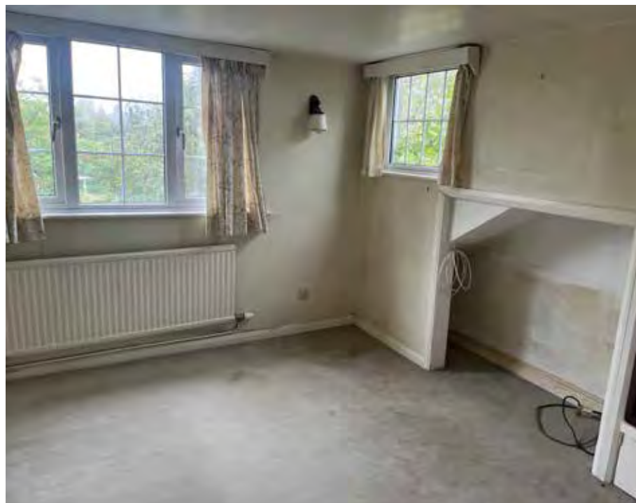
Internal view of Master Bedroom - Poor methods of construction & damp | 2025
