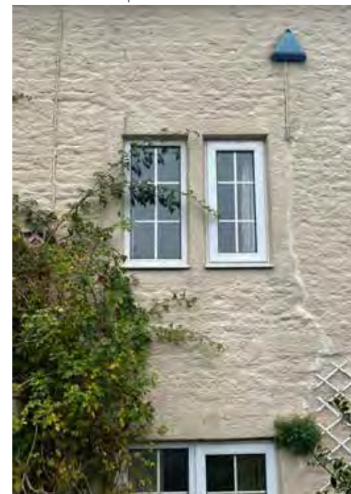
External view of front elevation - Ongoing structural movement | 2025
