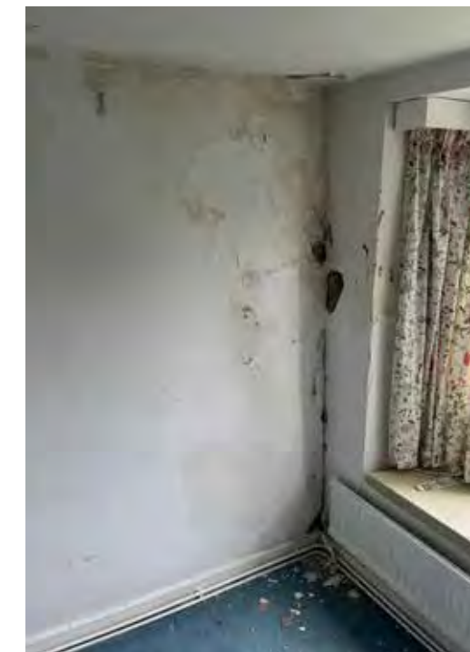
Internal view of first floor Bedroom One - Structural movement & damp | 2025
