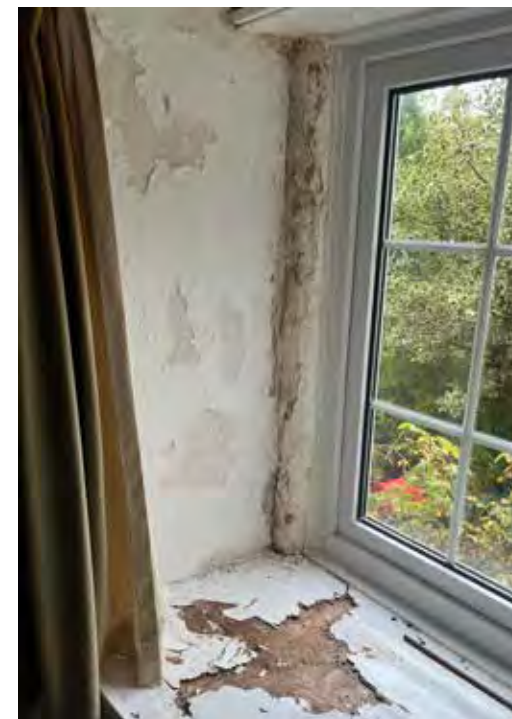
Internal view of first floor Bedroom Two - Structural movement & damp | 2025
