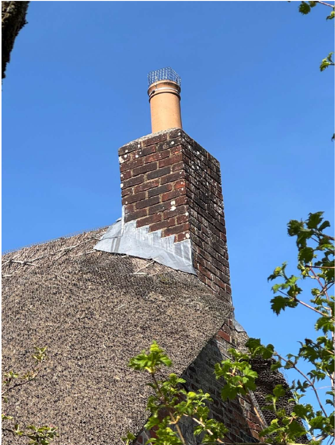
Close up Right Stack
