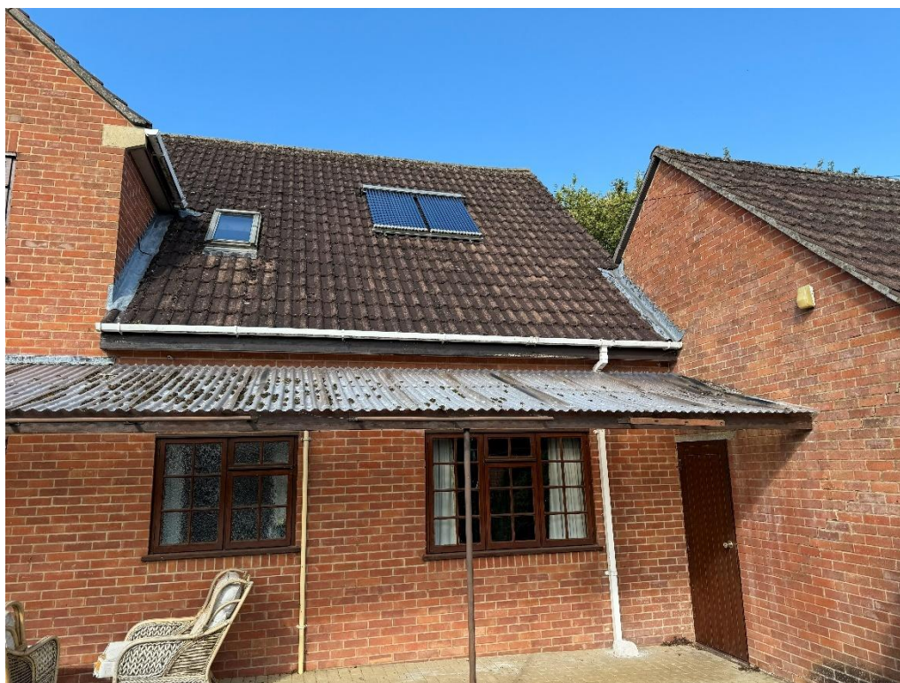
Figure 7 - Rear elevation showing evacuated tubes for water heating
