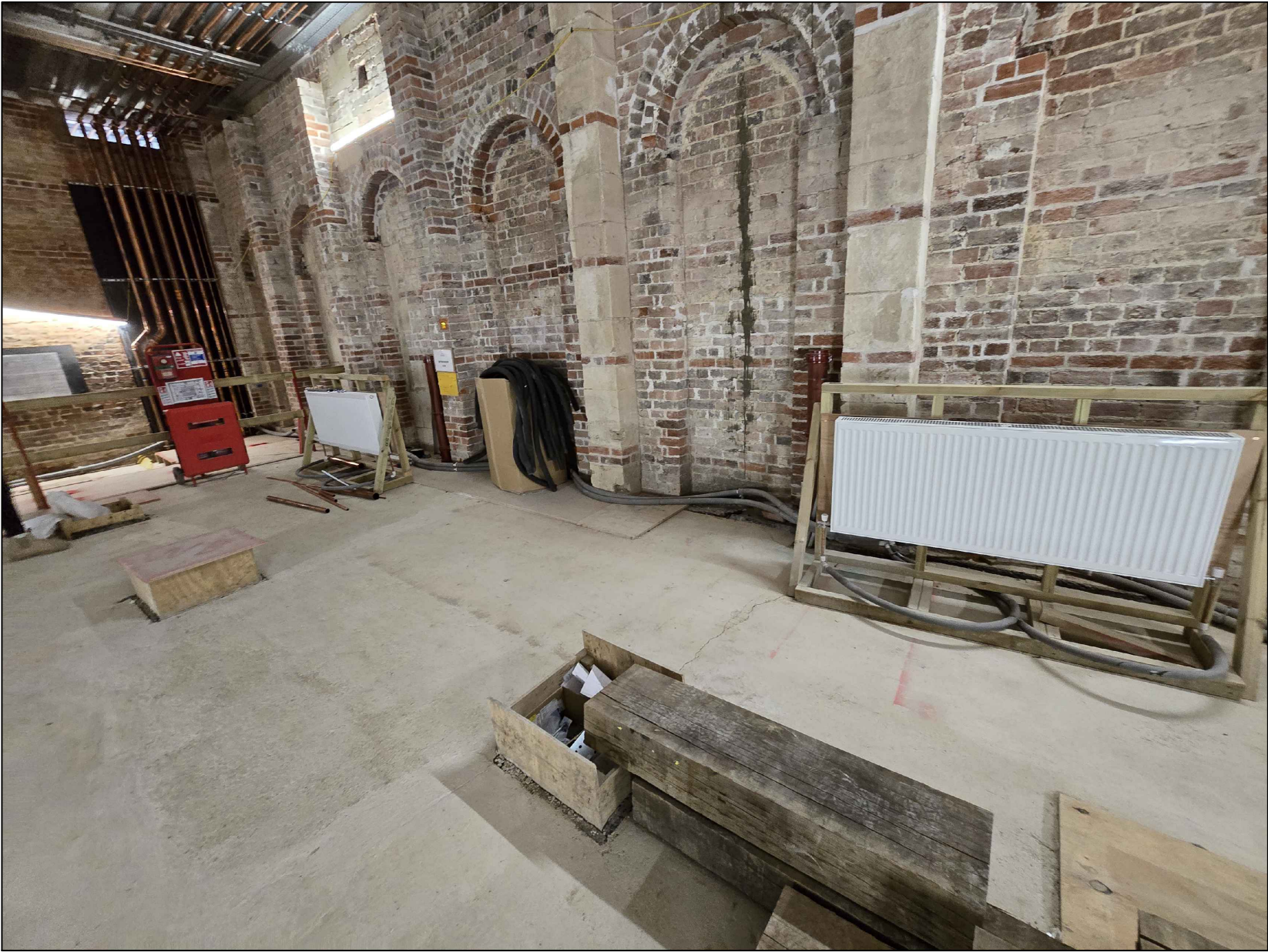
6 - Ground Floor - Limecrete Cracking
