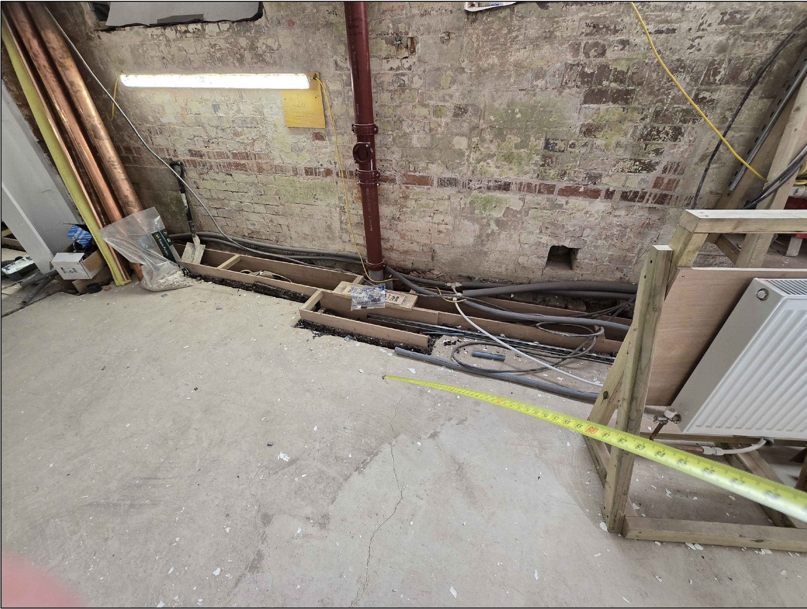
4 - Ground Floor - Limecrete Cracking
