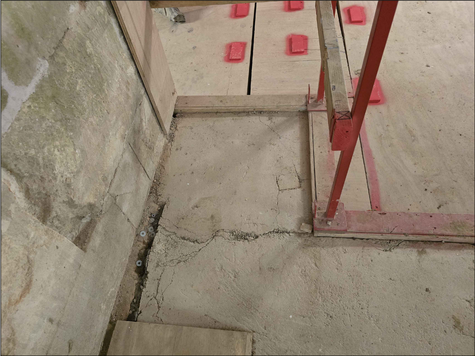
3 - Ground Floor - Limecrete Cracking
