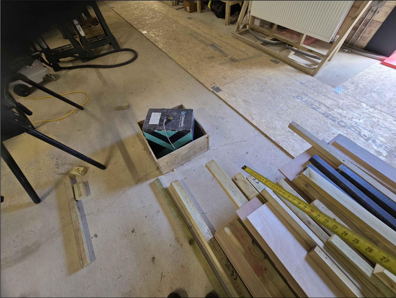
1 - Ground Floor - Limecrete Cracking
