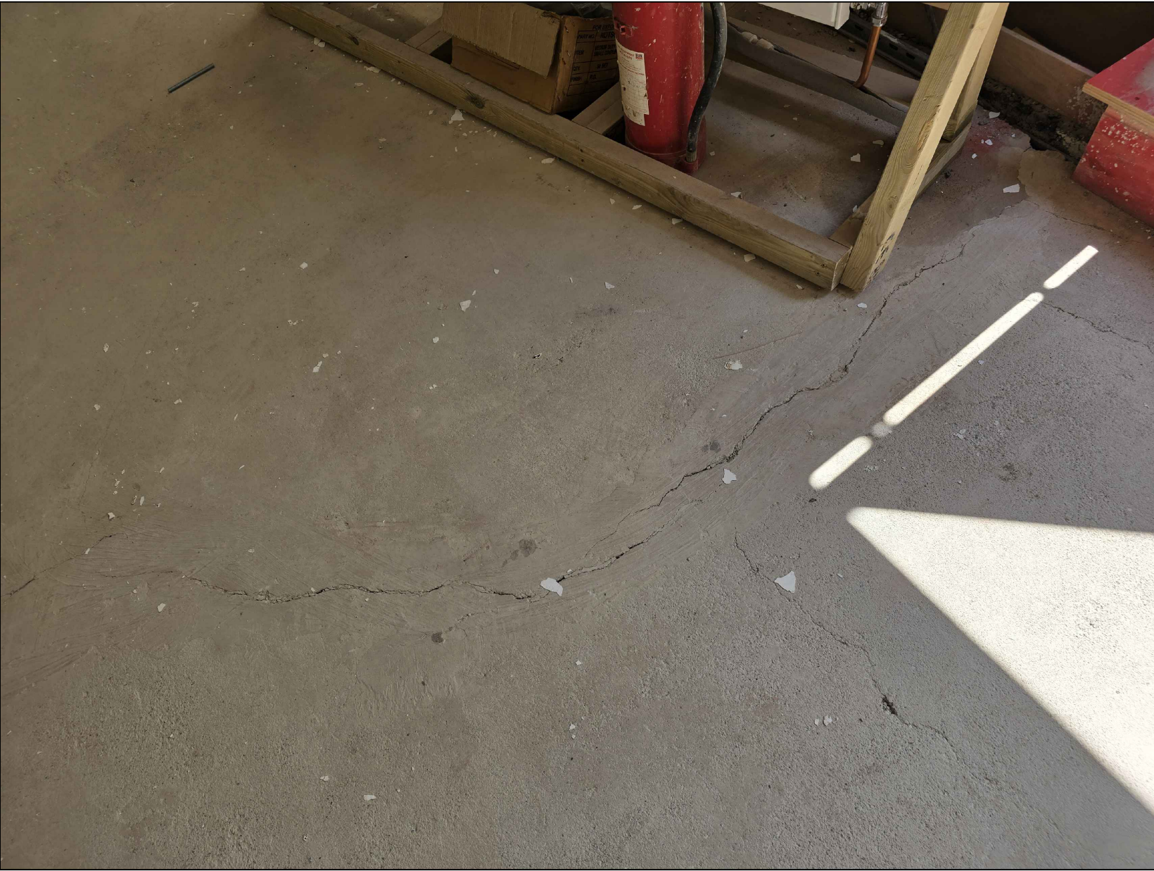
5 - Ground Floor - Limecrete Cracking
