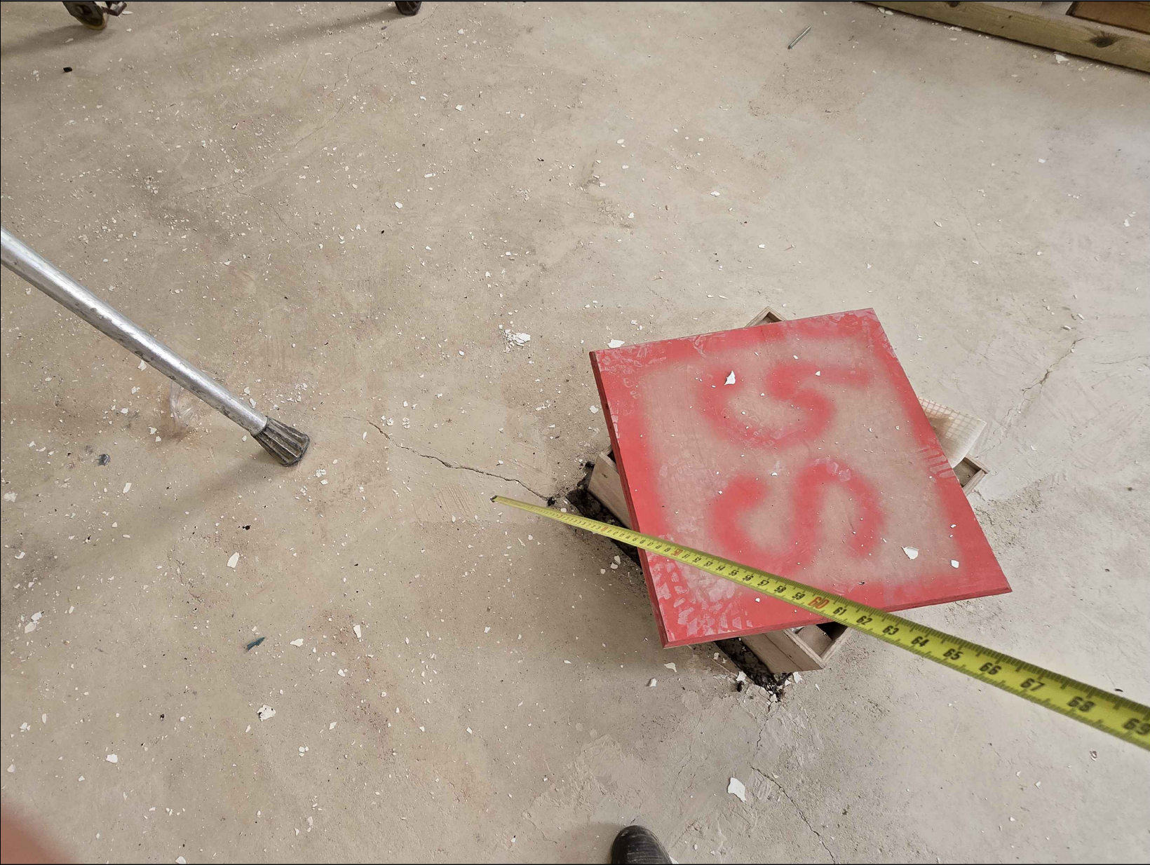
2 - Ground Floor - Limecrete Cracking
