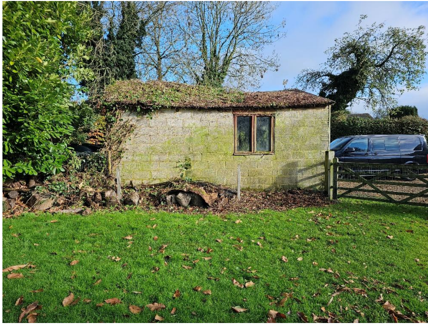
Figure 4 – West Elevation of the existing dilapidated garage building
