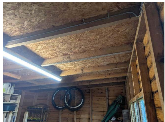
Photo 6 – internal view of shed showing no PRF's
