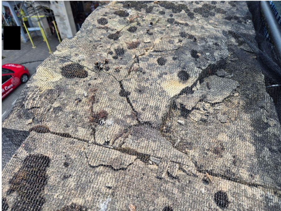
View of the damage to the parapet copings to the North East elevation and protective netting fitted over.
