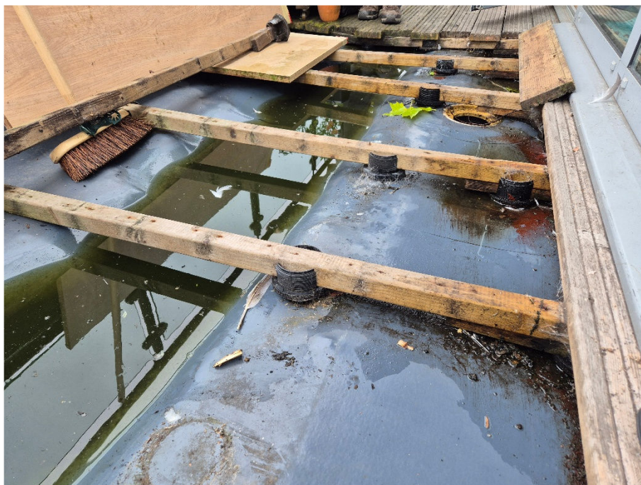
View of the roof terrace deck. Note standing water to partially collapsed sections.
