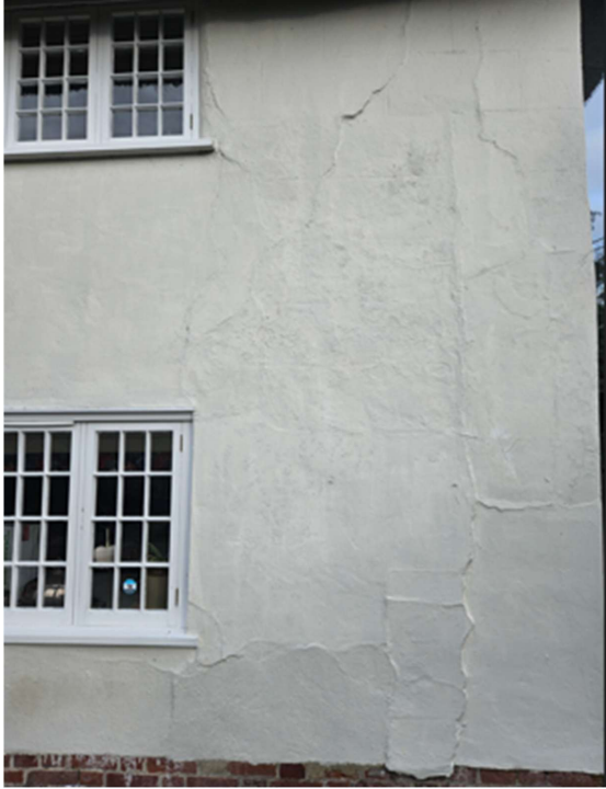
Examples of delamination, cracking and Ivy penetration:
