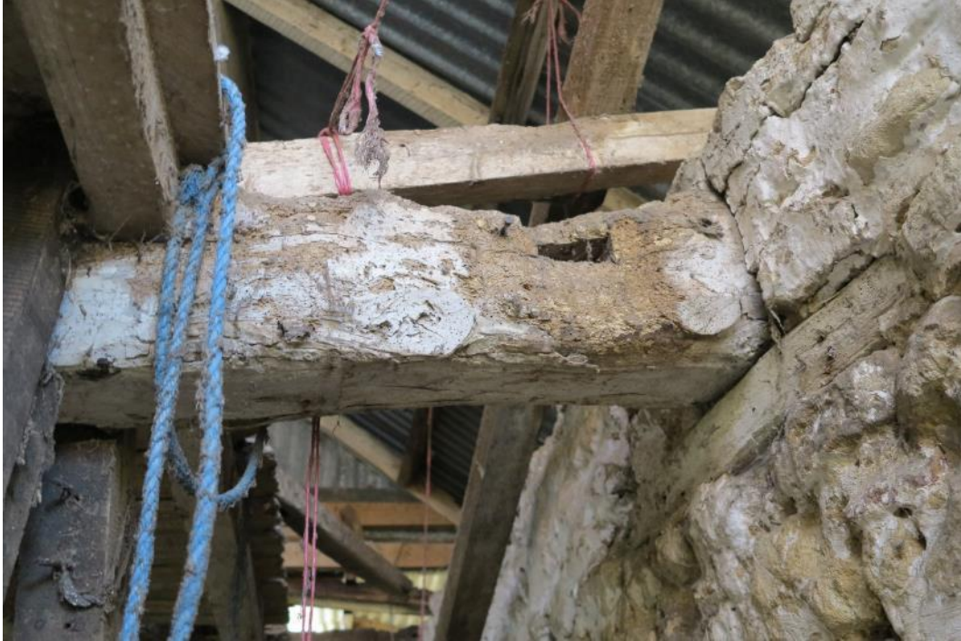
Plate 23. The damaged end of the transverse beam at the northern end of Structure 1; note the modern plank roof structure visible beyond
