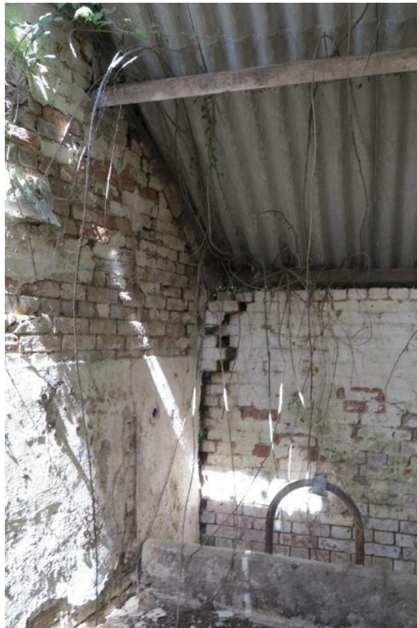
Plate 46. The rear wall of structure 4 is coming away from the south-western gable elevation
