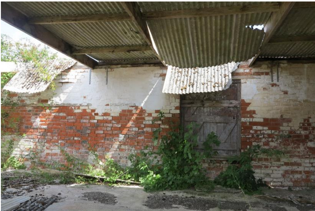
Plate 28. The modern flat roof in the main range of structure 1 is failing
