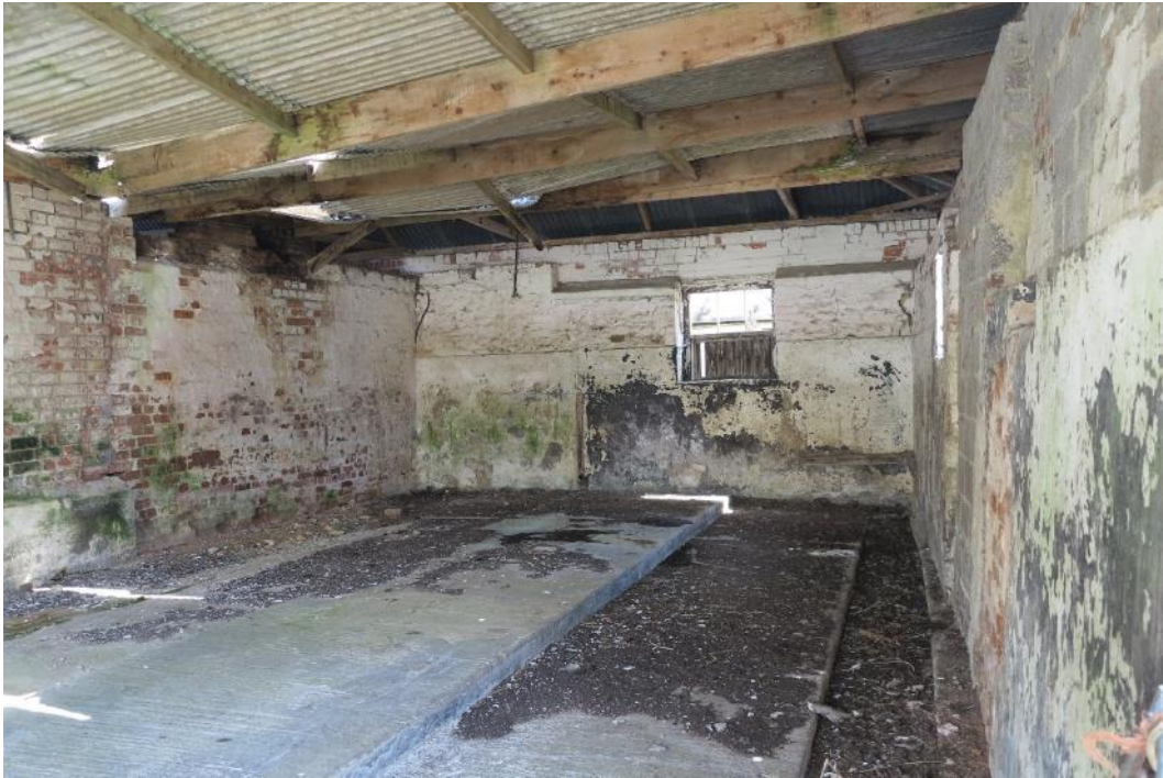
Plate 29. The modern flat roof in the main range of structure 1 is failing
