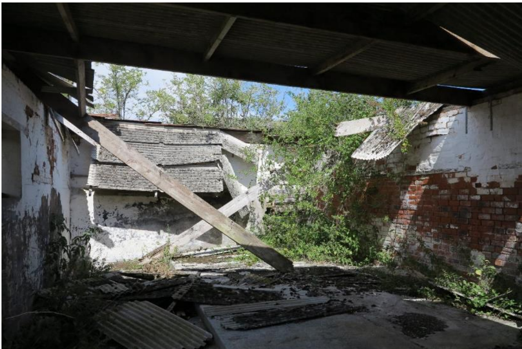
Plate 30. The modern flat roof in the main range of structure 1 is failing
