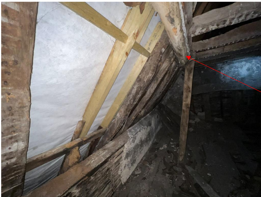
Photograph 04 7 and 9 Fish Row, Salisbury SP1 1EX Room 9 – Facing North – Showing propped fractured purlin
