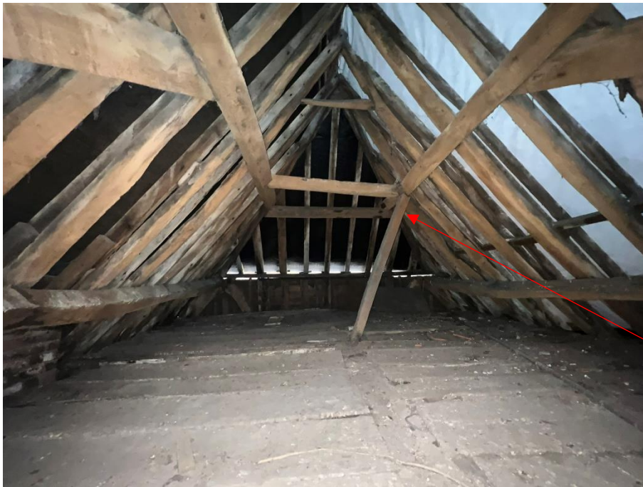
Photograph 01 7 and 9 Fish Row, Salisbury SP1 1EX Room 11 – Facing South – Showing propped fractured purlin
