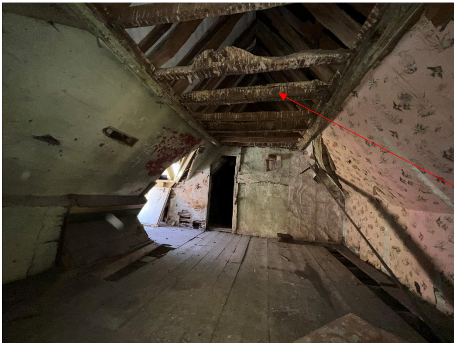
Photograph 02 7 and 9 Fish Row, Salisbury SP1 1EX Room 10 – Facing North – Showing deteriorated ceiling ties
