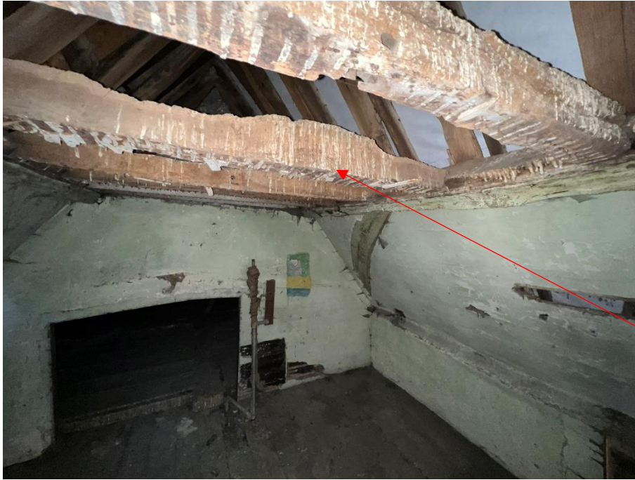
Photograph 03 7 and 9 Fish Row, Salisbury SP1 1EX Room 10 – Facing South – Showing deteriorated ceiling ties
