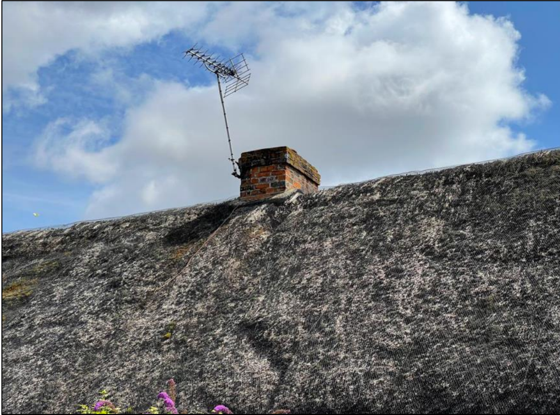
Manor Barn - eroded thatch covering and very short brick chimney.
