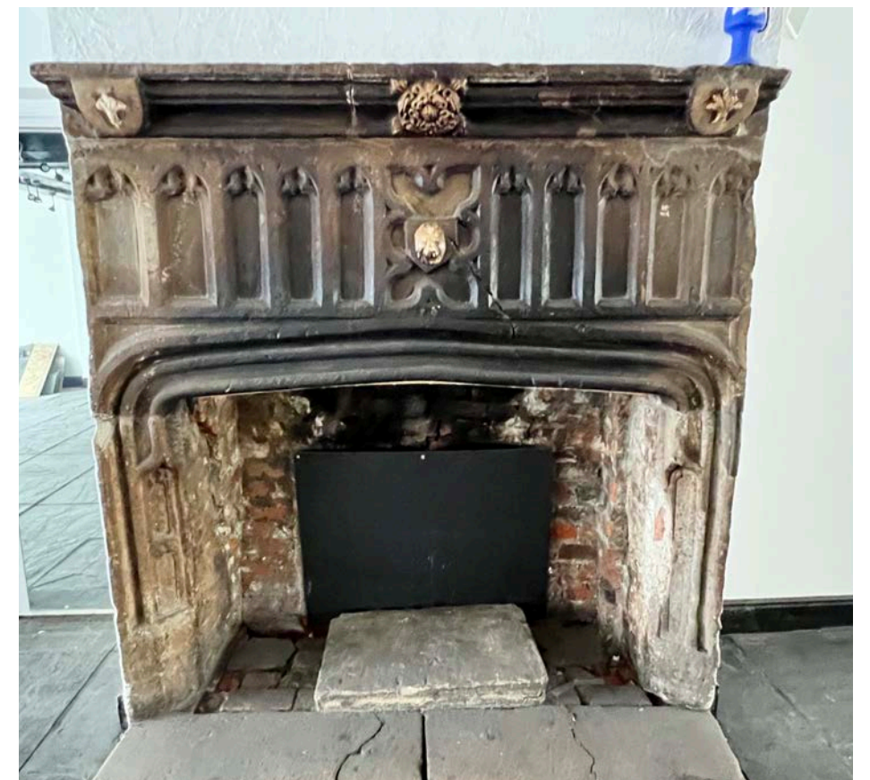
figure 24: 15th century fireplace to 7 Fish Row ground floor
