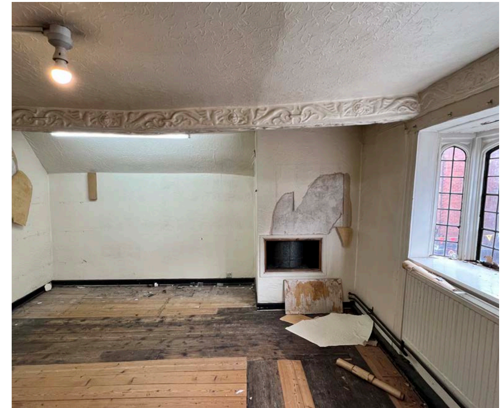
figure 33: second floor 17th century plasterwork and distorted beam which the Structural Engineer advises on investigation
