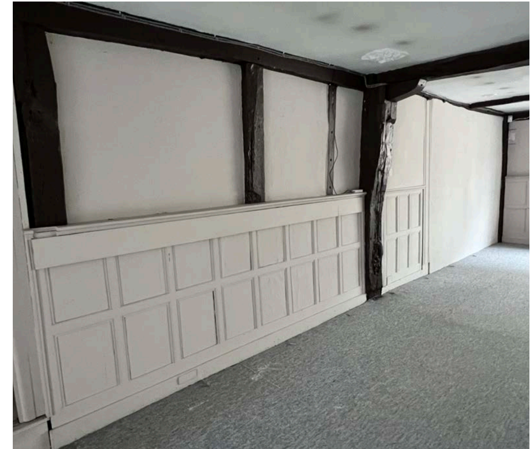
figure 31: 7 Fish Row first floor dado panelling reported as 19th century requires some repair and removal of modern rails,
