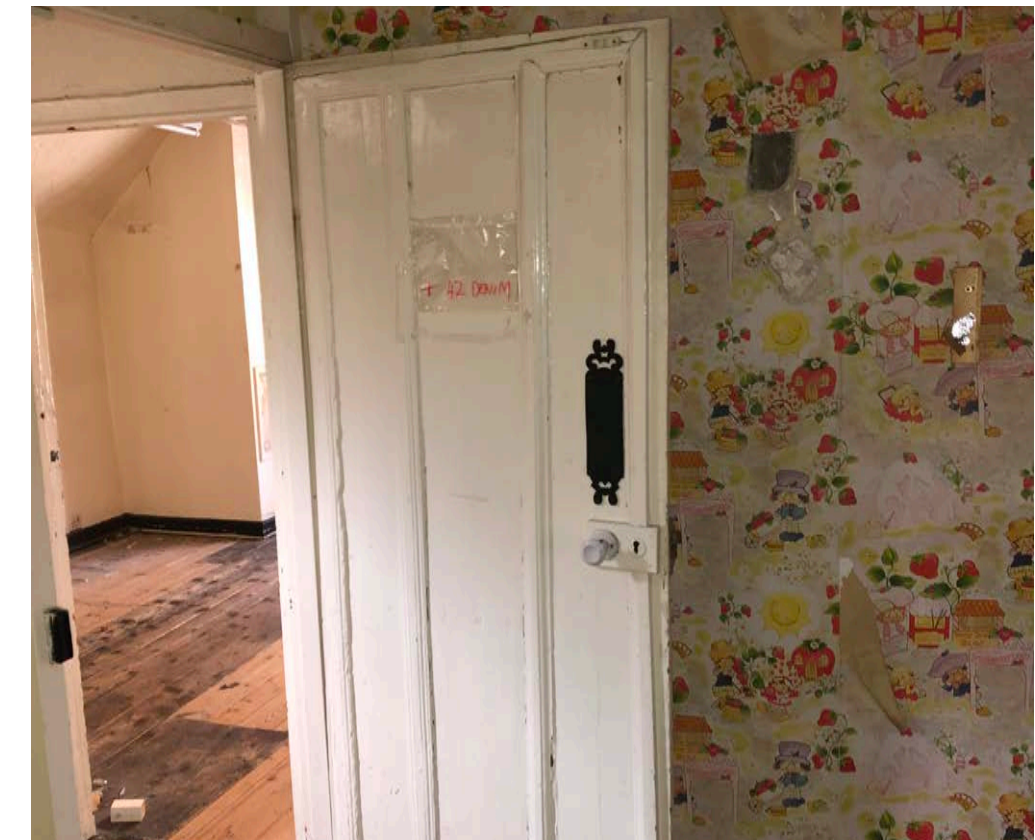
figure 34: 16th or 17th century door with original strap hinges to be retained and repositioned to avoid more intrusive fire upgrading.
