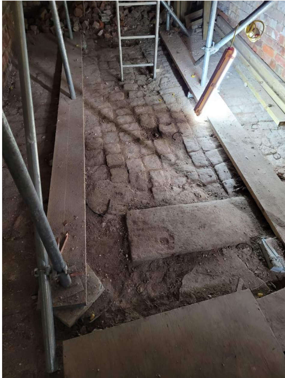
G10 - Stone setts in very poor condition
