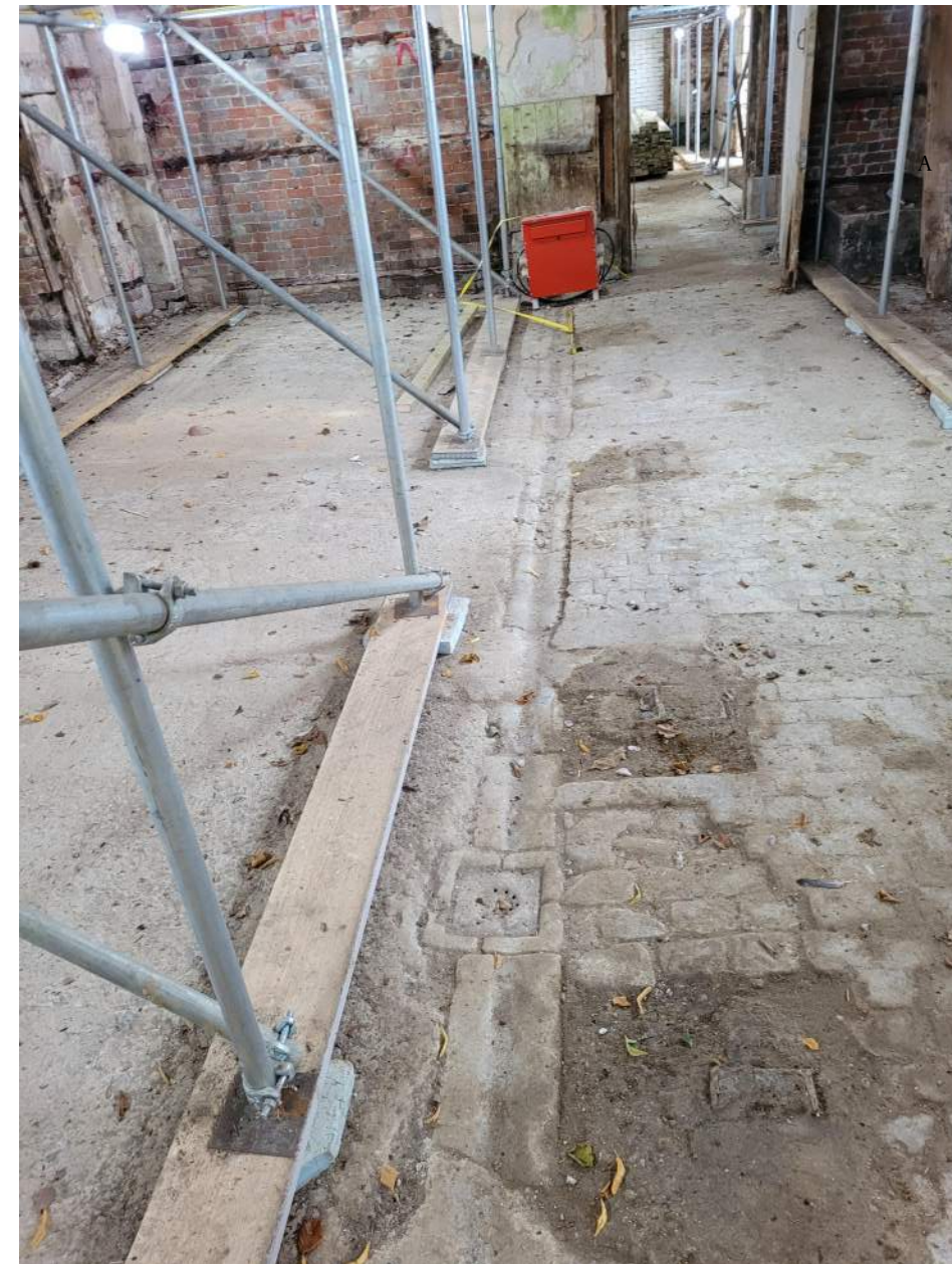
G24 - Mix of modern concrete and stone setts in poor condition
