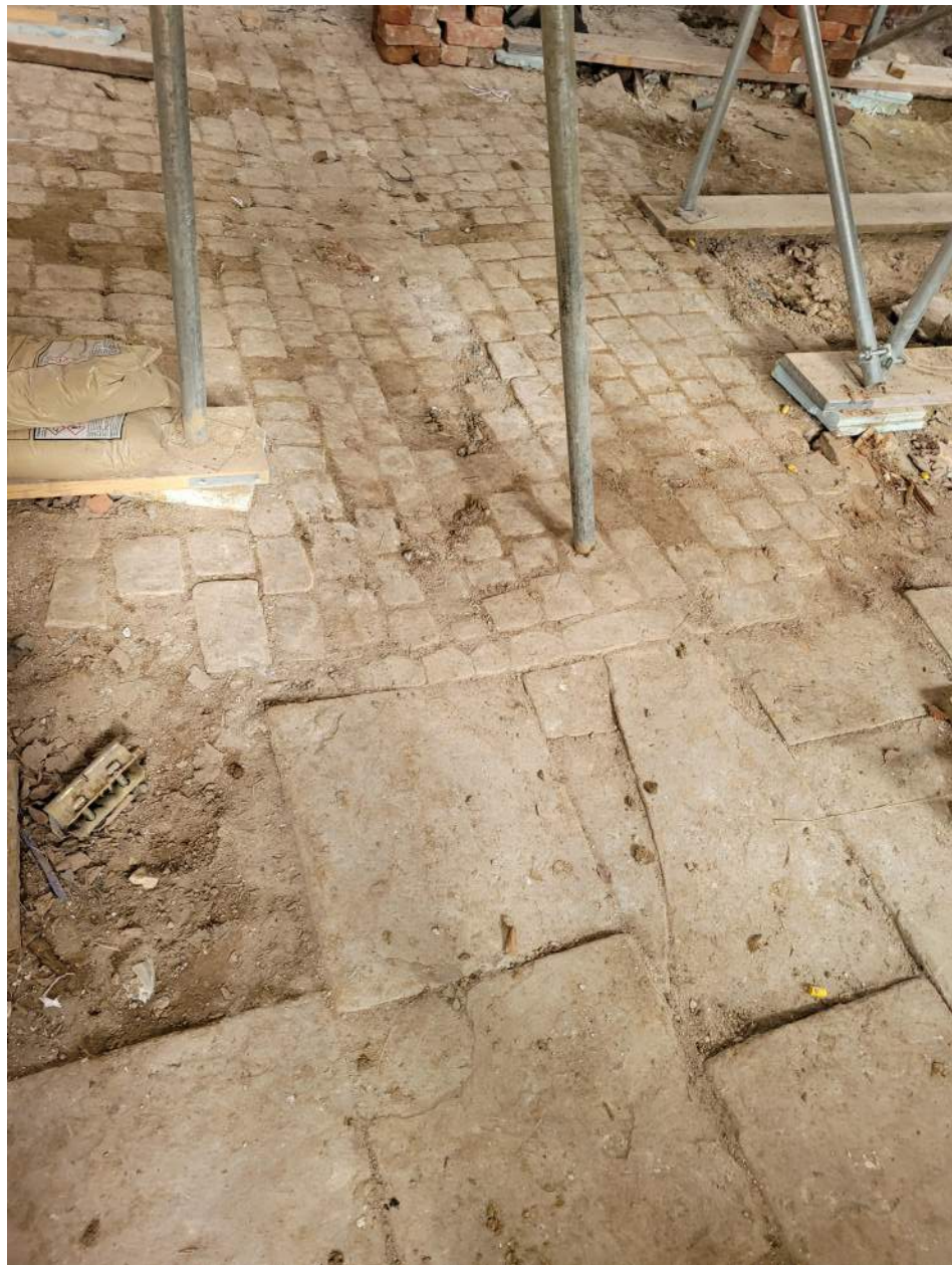
G12 - Mix of flagstones and stone setts in very poor condition
