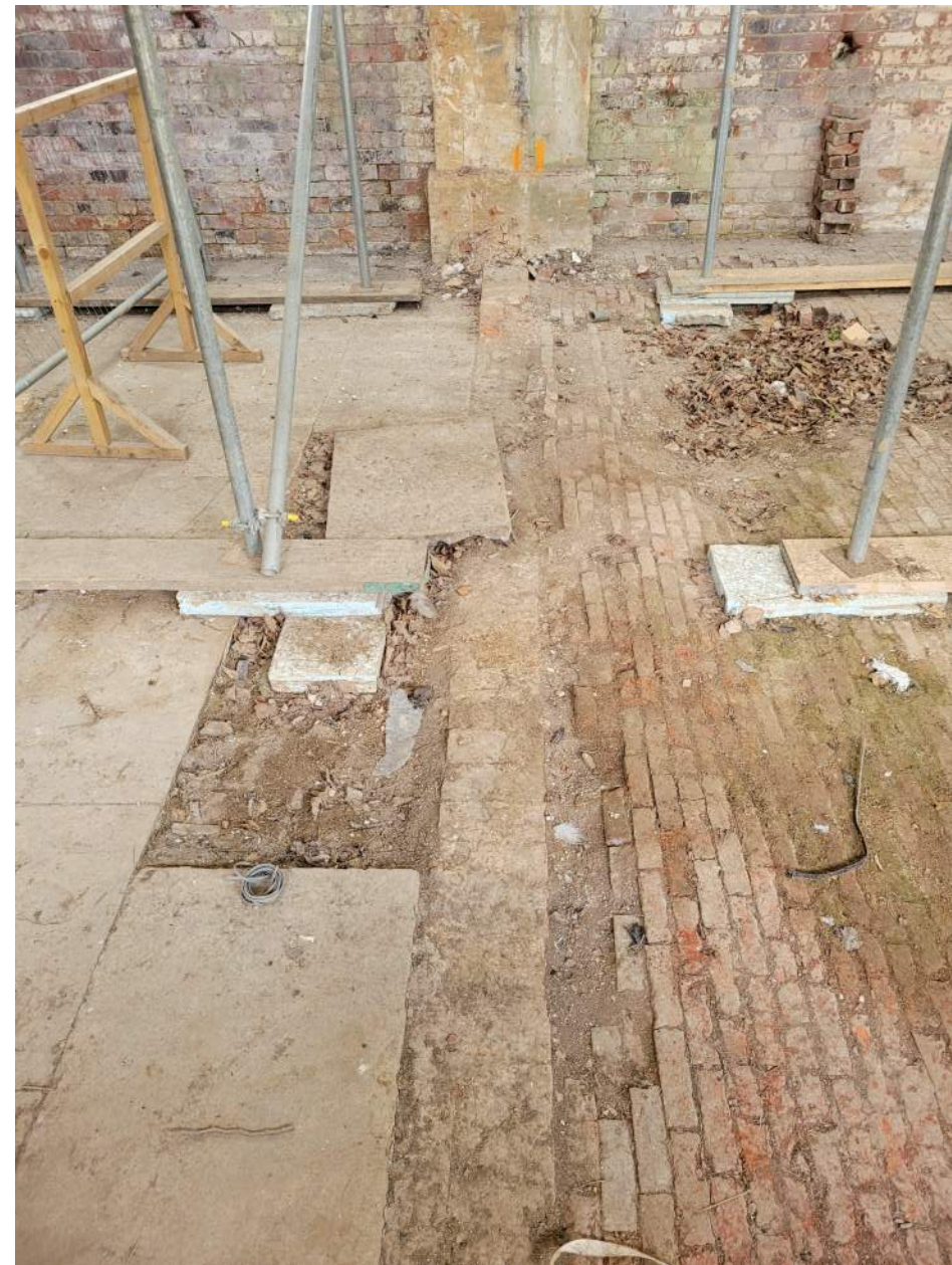
G20 & G21 - Mix of flagstone and brick in very poor condition
