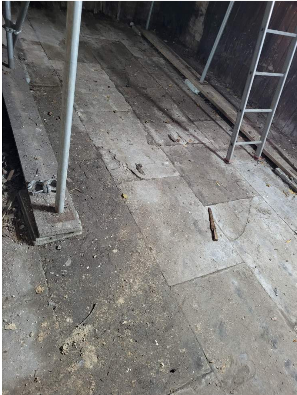
G02 - Flagstone flooring in poor/fair condition
