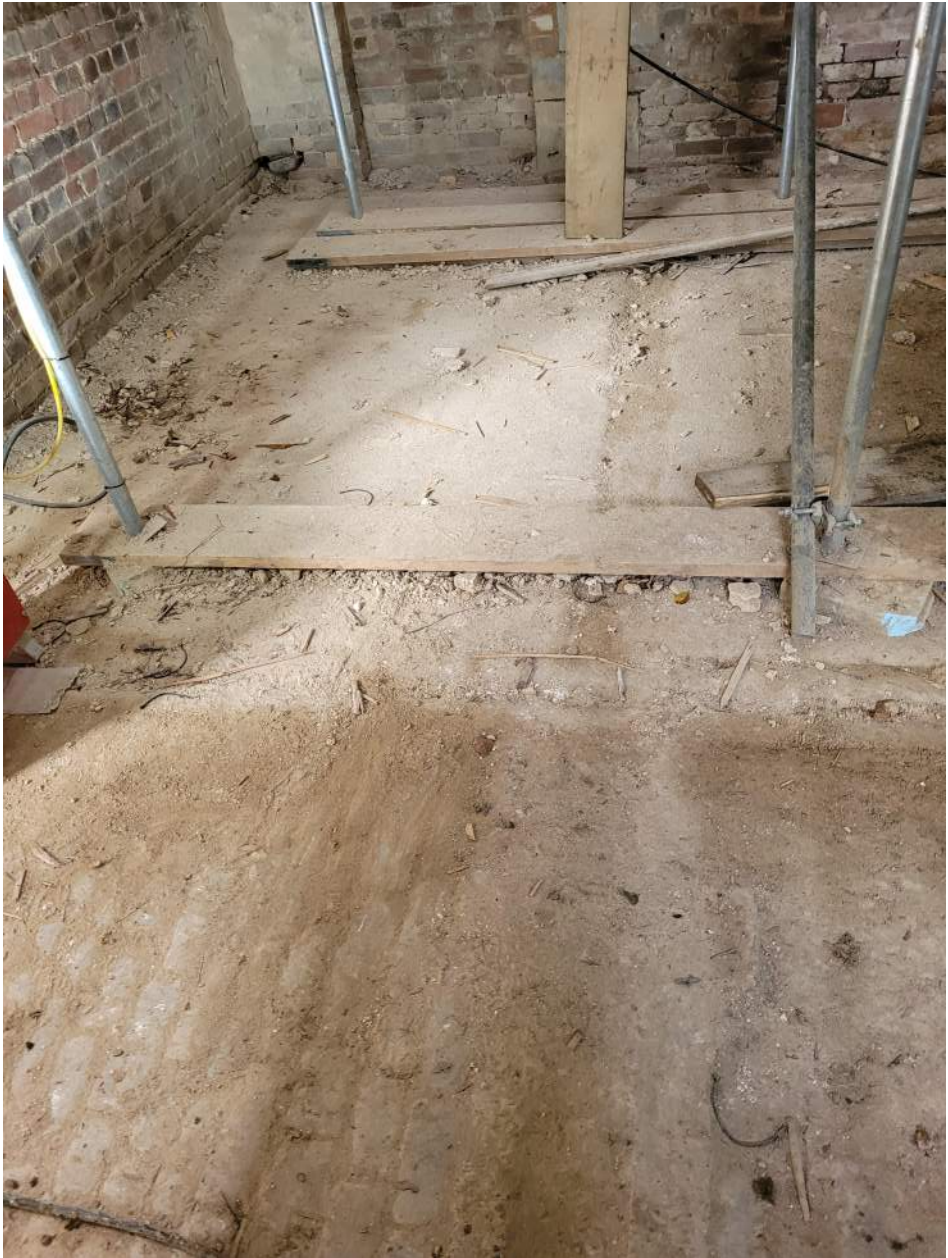
G06 -Mix of stone setts and modern concrete flooring in very poor condition
