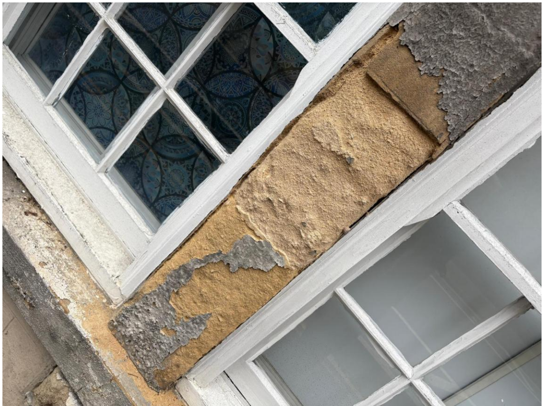
6. Significant erosion to stone window mullion – front ground floor.
