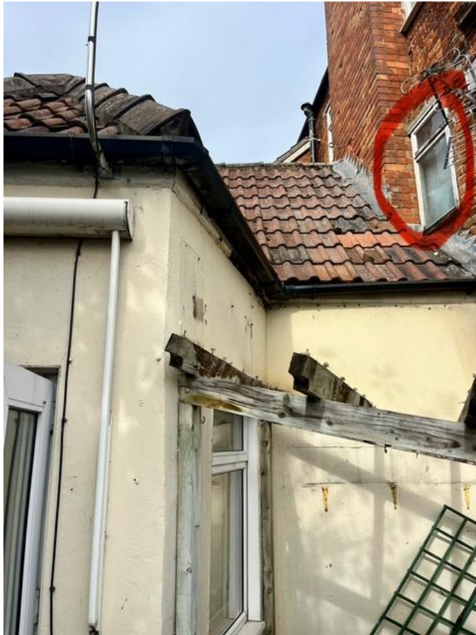
9. As above window to be replaced.
