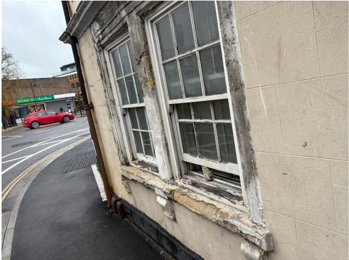
7. Significant erosion to window cill – front left hand side.
