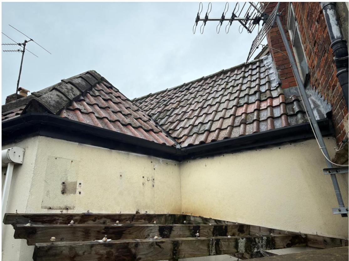
8. Decaying modern timber window requires replacement.
