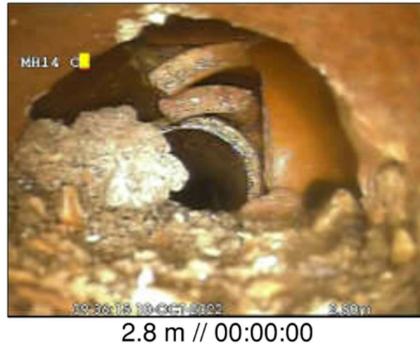
Figure 2 - CCTV Report showing existing foul water pipe junction with large joint displacement and excessive debris.
