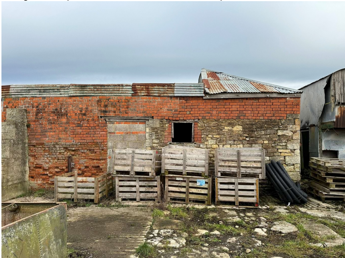
3 Longer view of photo 1 with the defective roof and the spalled low-level brickwork
