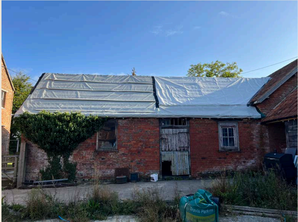
Figure 1: South Elevation of Stable 1 from courtyard showing temporary tarpaulin roof
