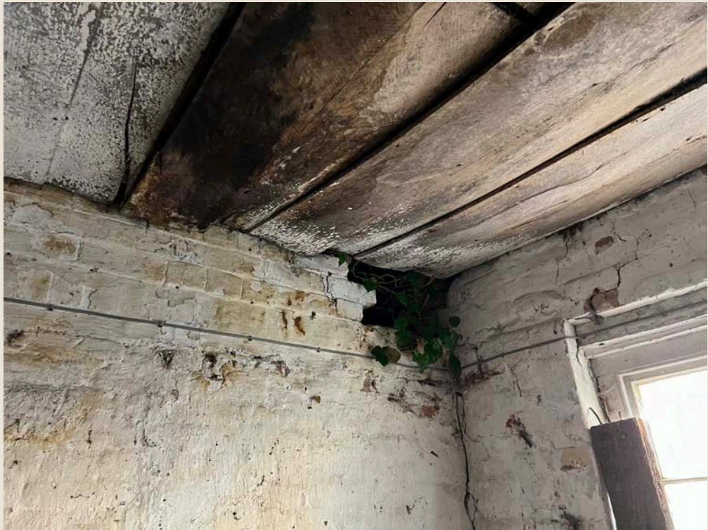
Figure 13: Stable 1 interior, water damage
