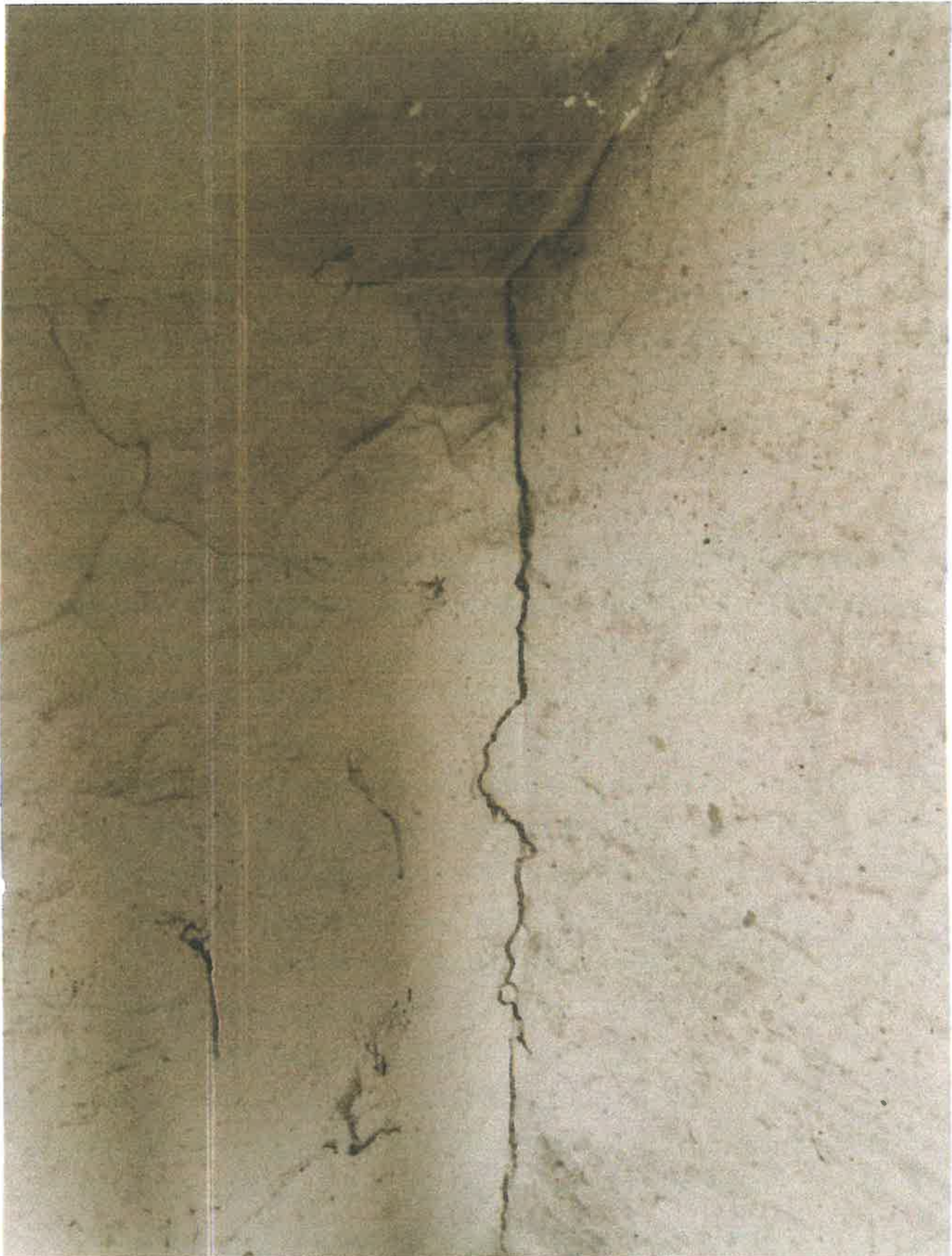
Figure 11 - Cracking down junction of walls and skeling of second floor.
