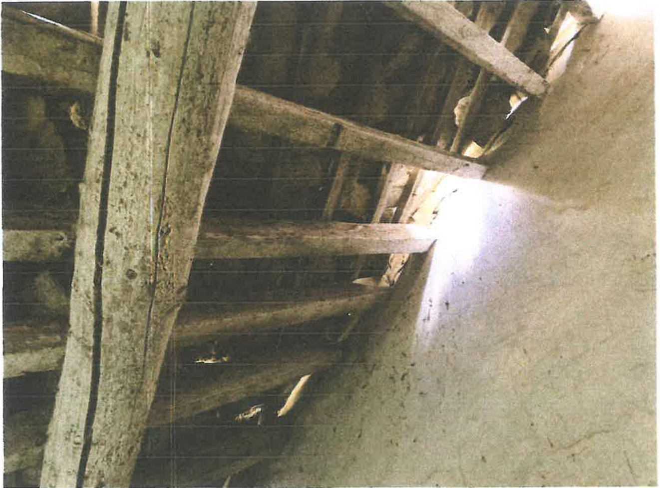
Figure 8 - Rafter junction of two storey mono-pitched roof to original building showing vertical slip of rafters down the face of the wall.
