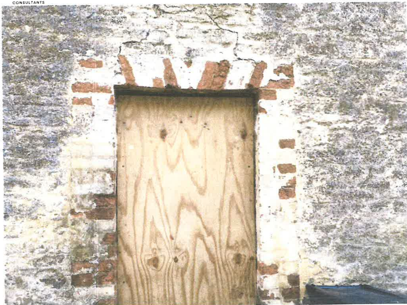
Figure 7 - Frost damage to brickwork feature limb and revealed, along with cracking to stone above limb.
