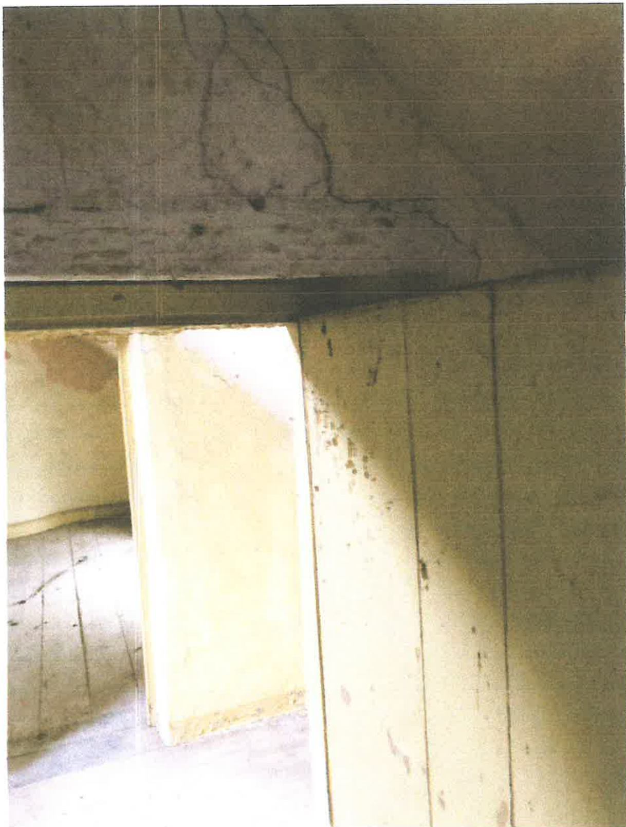
Figure 1 - Cracking over internal door lintel at second floor spine wall of the original property
