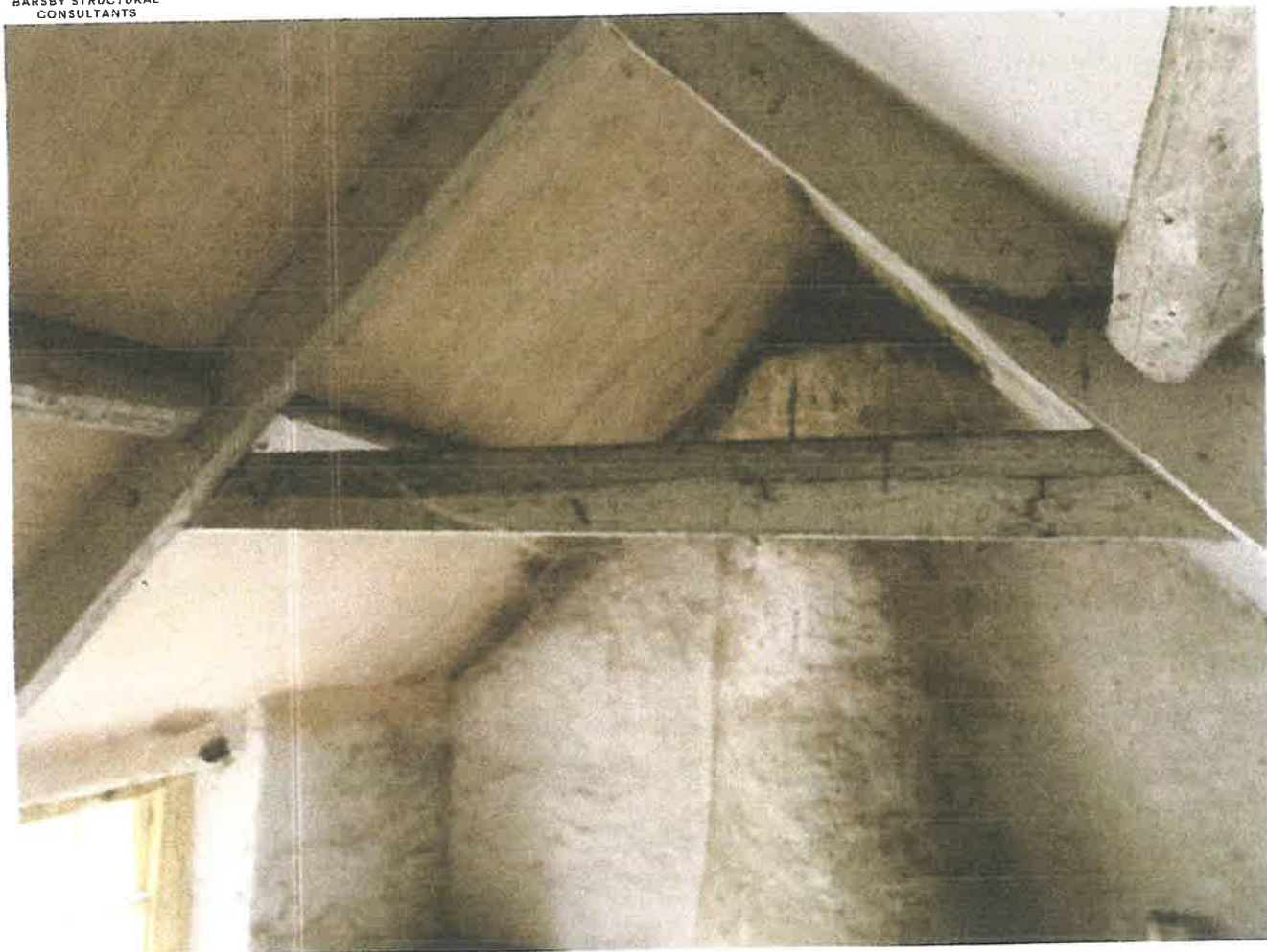
Figure 10 - Eastern half of main roof showing truss and missing ceiling collars.
