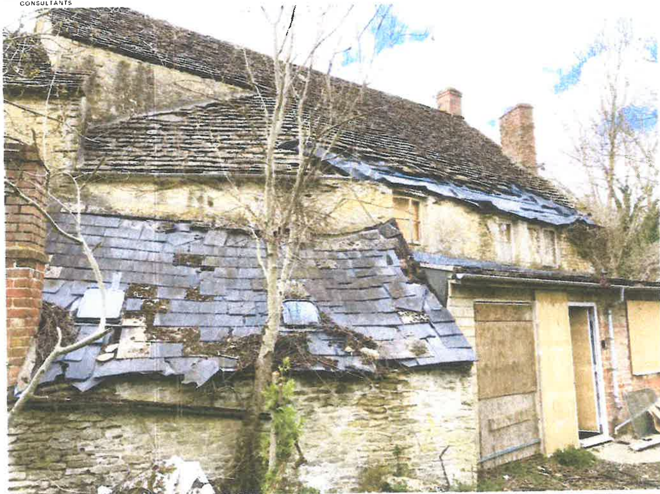
Figure 5 - Rear elevation showing poorly constructed single storey extensions and missing roof tiles.
