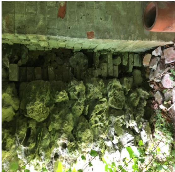
Fig 10: Collapsed brickwork at Western arch.
