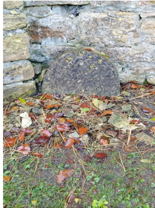
Fig 15: Dislodged merlon end cappings to be reinstated.
