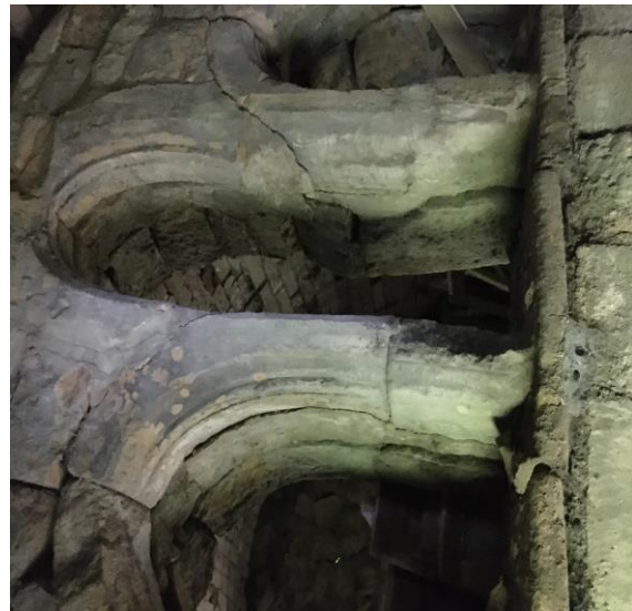
Fig 11: Fractured/collapsed stonework to internal windows.
