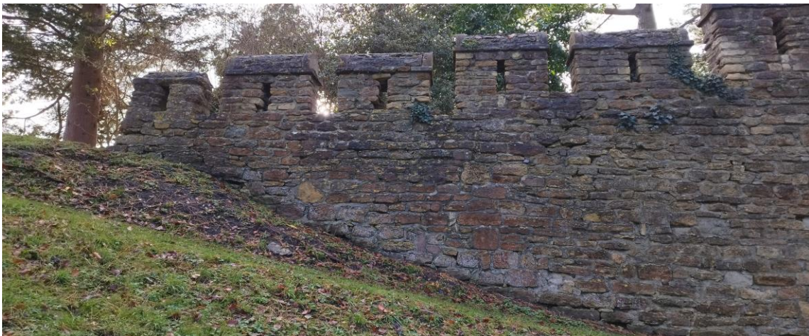
Fig 17: Areas of cement mortar pointing on East Elevation to be raked out and repointed using lime-based mortar.
