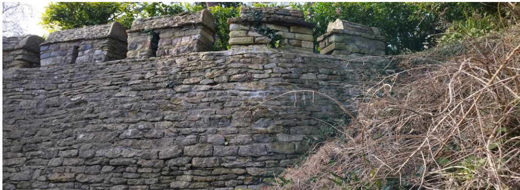
Fig 16: Areas of cement mortar pointing on East Elevation to be raked out and repointed using lime-based mortar.
