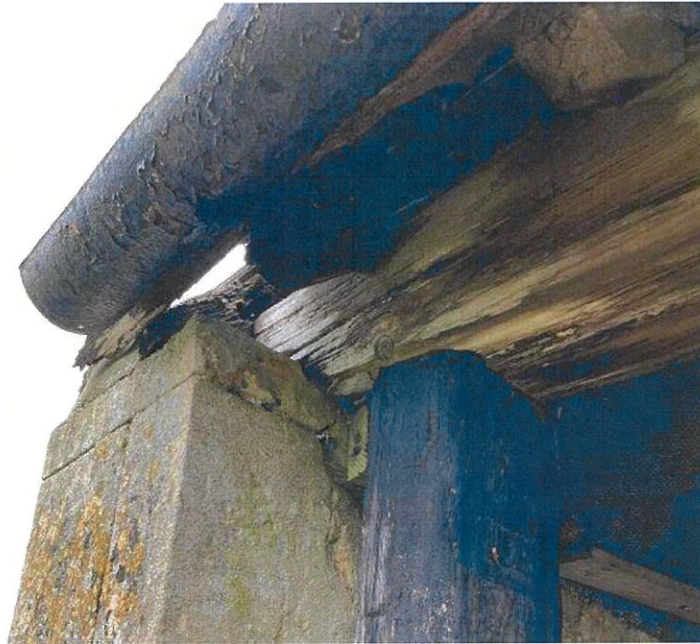
9. Decay at West End of Eaves Beam
