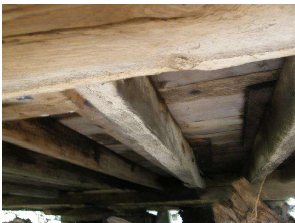
Fig.58 Underside of granary
