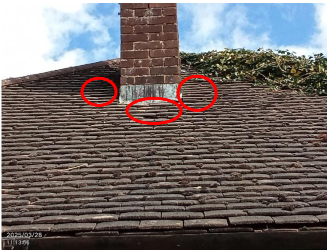
Photo 4: Raised tiles around the chimney on the west elevation.
