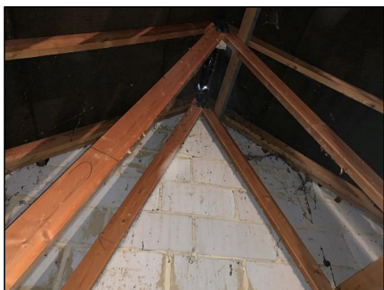
Photo 9 Loft void gable end with bat droppings
