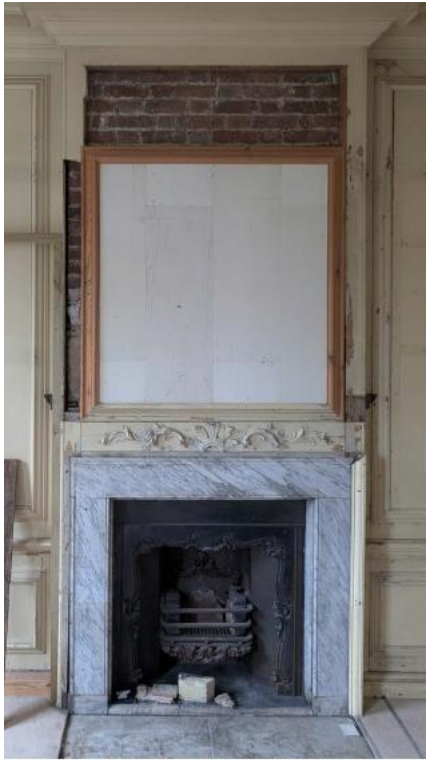
Fireplace, with displaced modern panel above and missing mantle shelf
