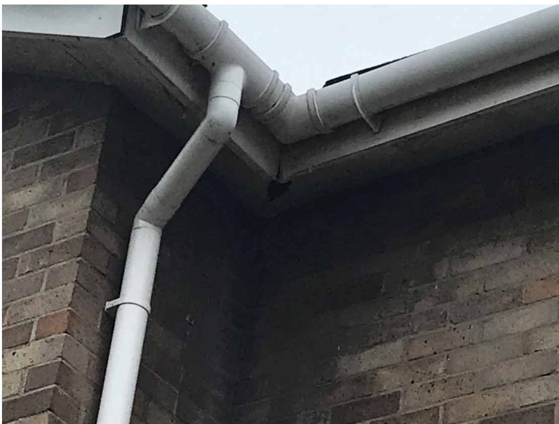
Photograph 5: B1; west wing; south-west aspect. Hole in the soffit visible.
