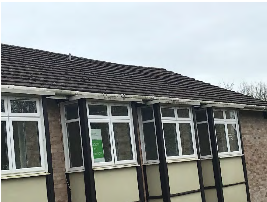
Photograph 4: B1; south-east wing; north-west aspect; view from the north. Gap under the end ridge tile visible.
