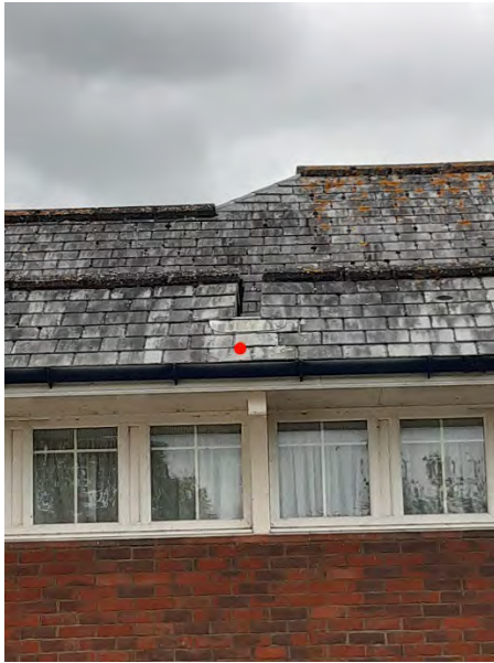
Photograph 4: Braemar Lodge roof showing lifted tile (marked by red dot).
