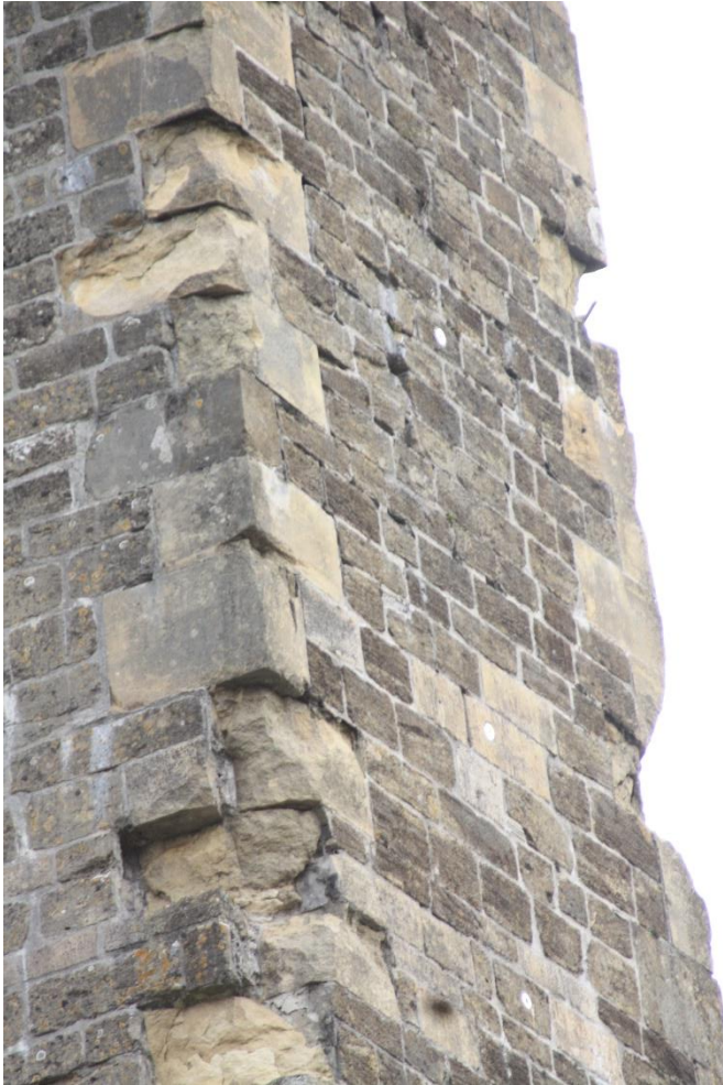
Figure 5 Detail of the damage to masonry on the south-west face of the main shaft of the monument
