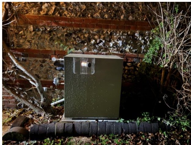
Installed Replacement Oil Boiler (2025).
