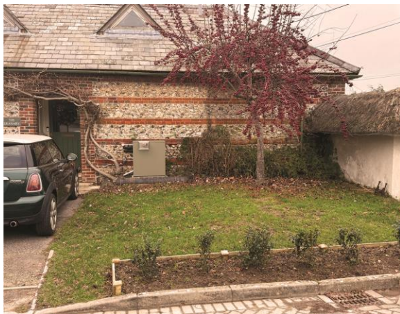
Existing Photo of Boiler Currently Installed
