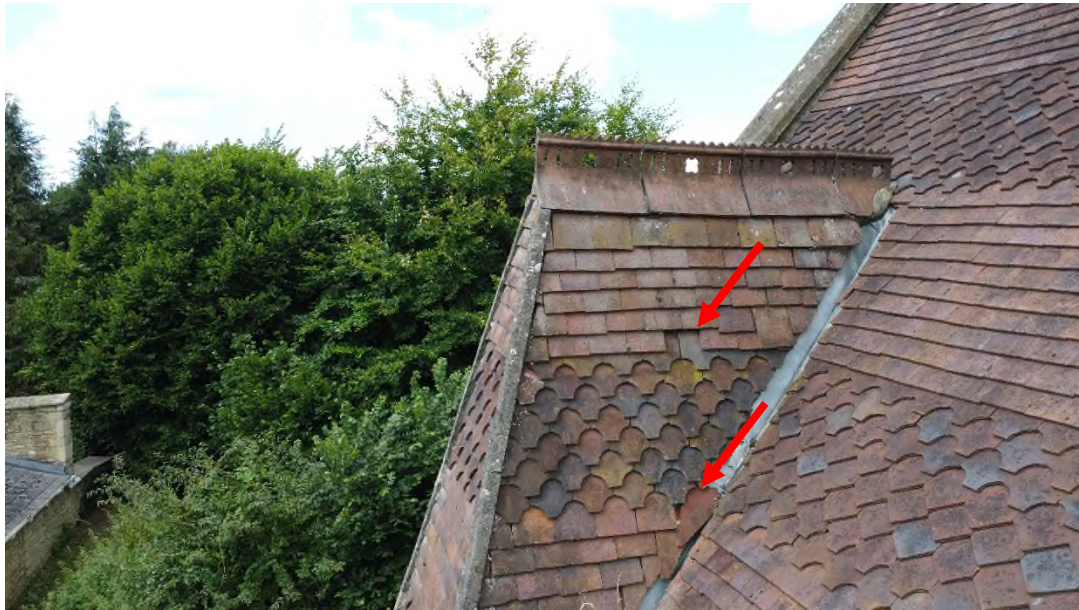
Plate 7 slipped tiles on the roof potential for birds and bats, but no evidence of use
