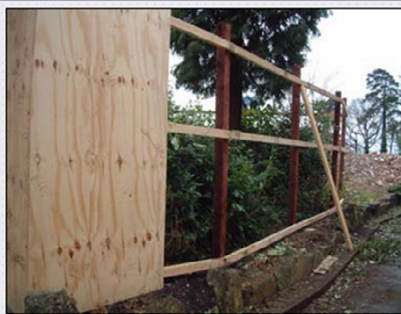
Board specification on secure wooden posts
