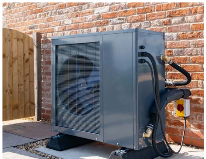
Air source heat pump (ASHP) provision
