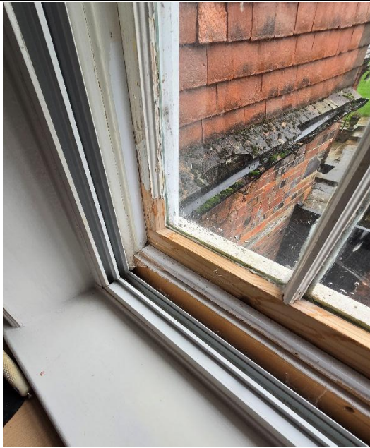
F4 Lower sash left-hand corner
