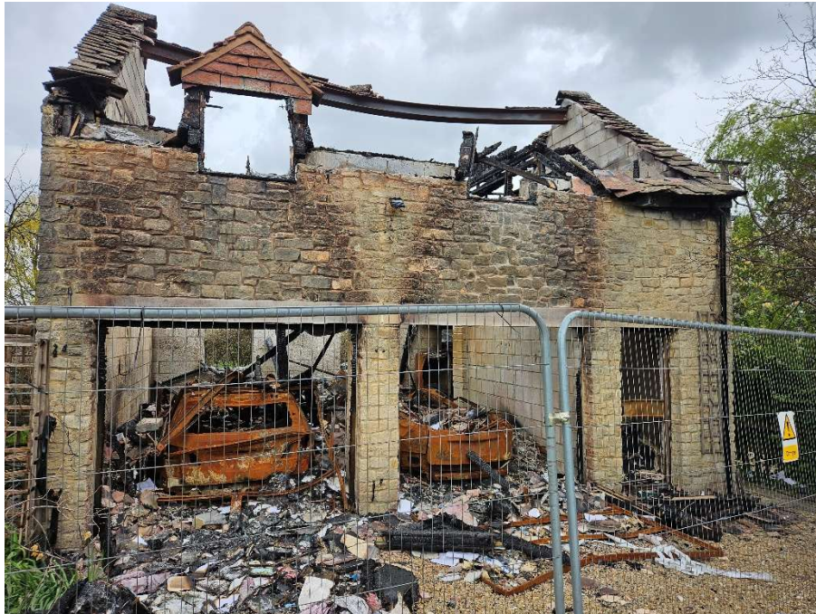
Photo 1 – South (Front) Elevation – Post Fire
