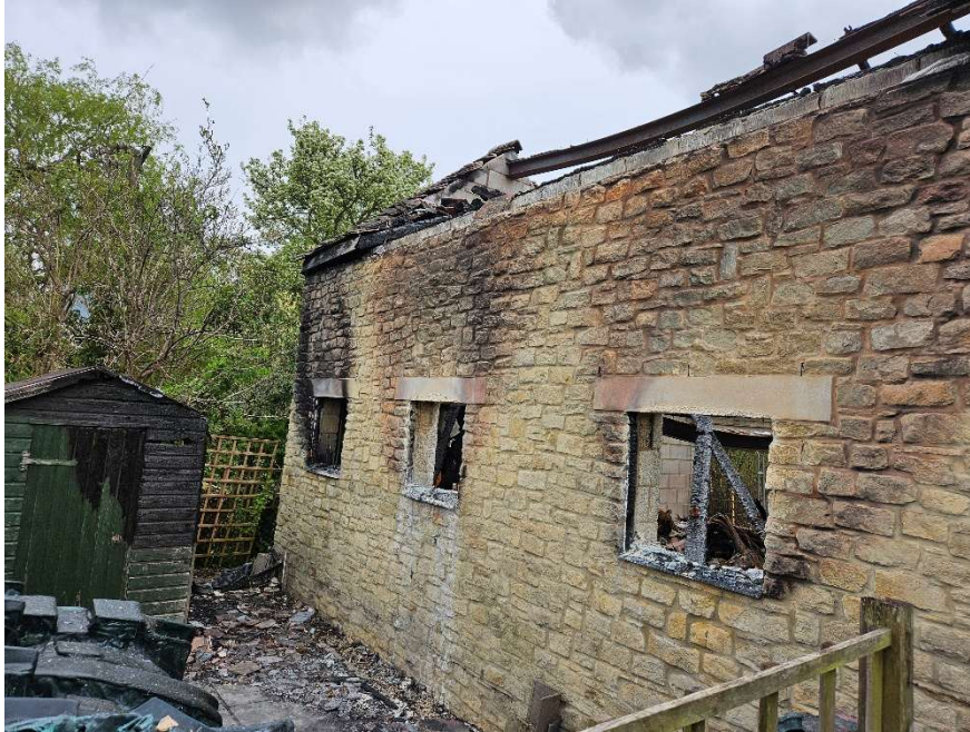
Photo 3 – South (Rear) Elevation – Post Fire
