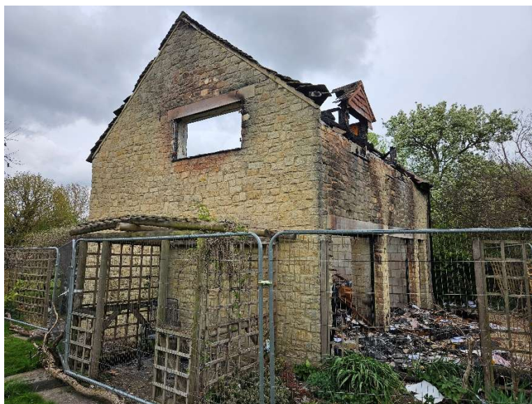
Photo 2 – West Side Elevation - Post Fire
