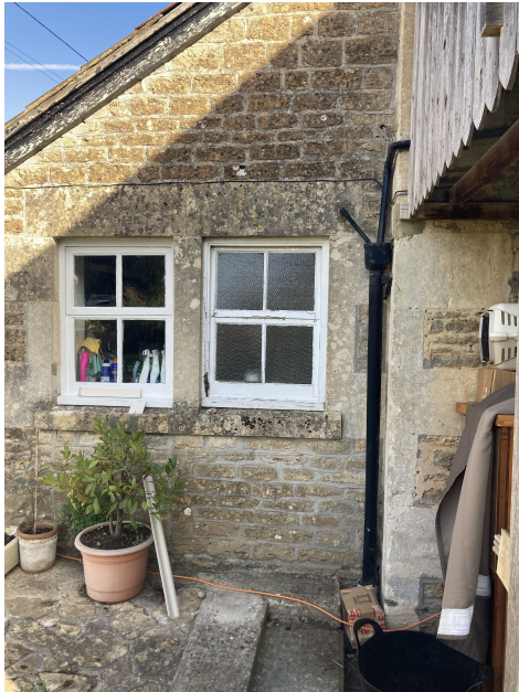
photo showing G-W-15&16. Window to match as close as practical
