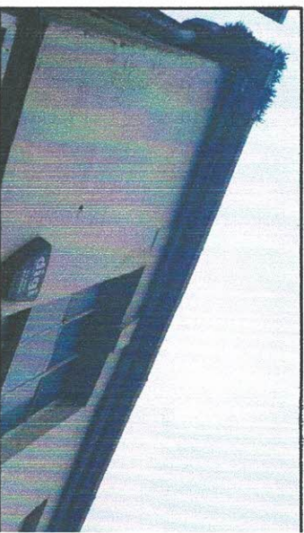
Photo 5 B1 and B2 gap under roof edges
