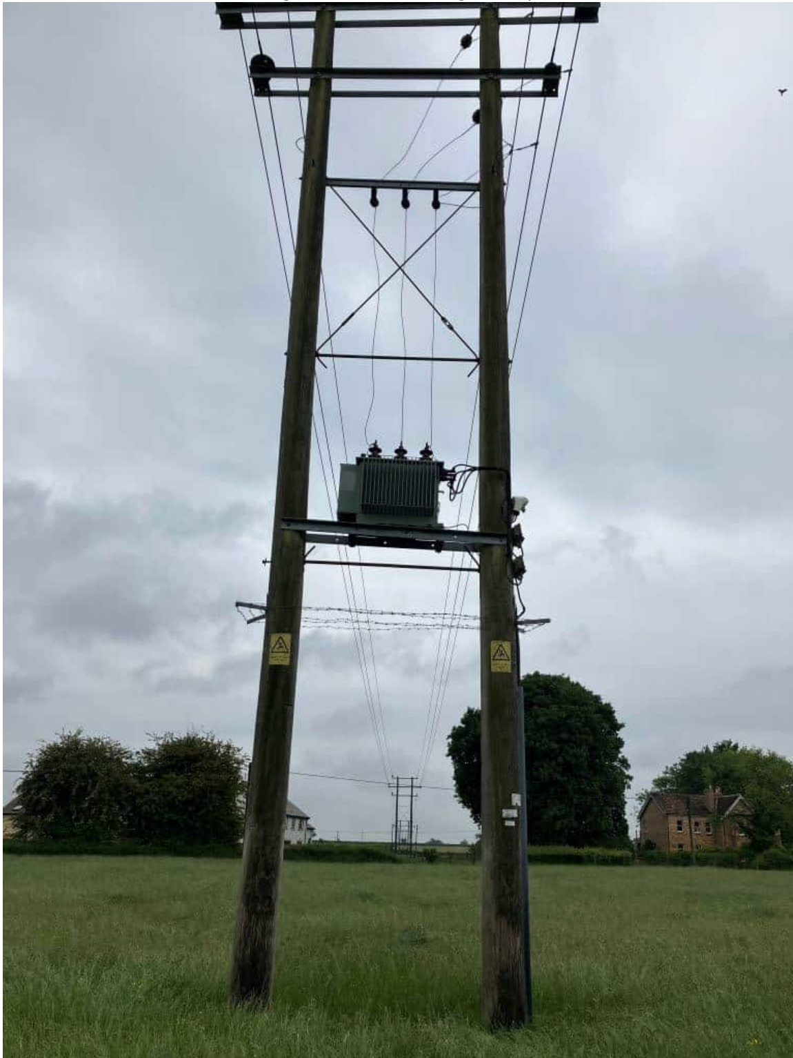
Photograph 19 – Pole mounted electricity transformer associated with the overheads running through Site.
