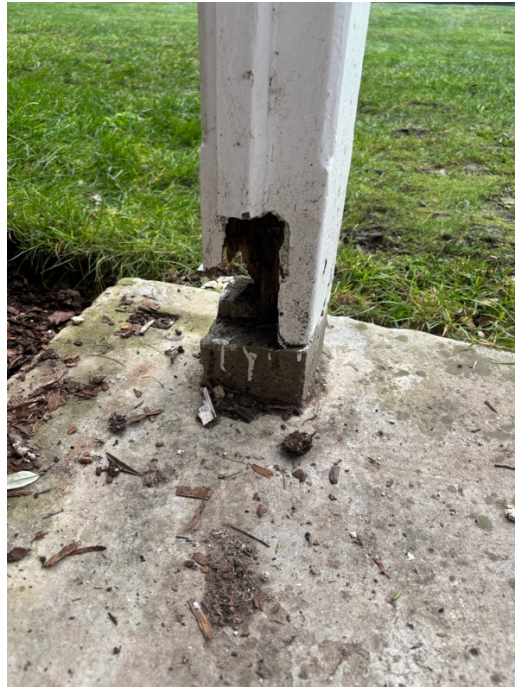
Existing rot to posts
