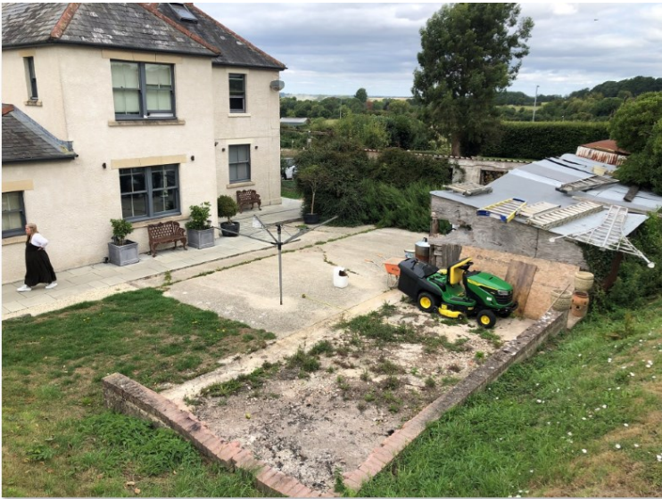
West Facing Dilapidated Outbuildings
