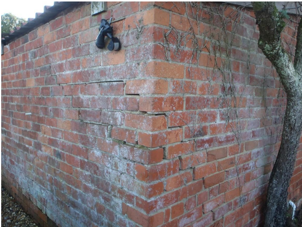
Photograph 6: showing gaps in the wall of Section 3 of the building
