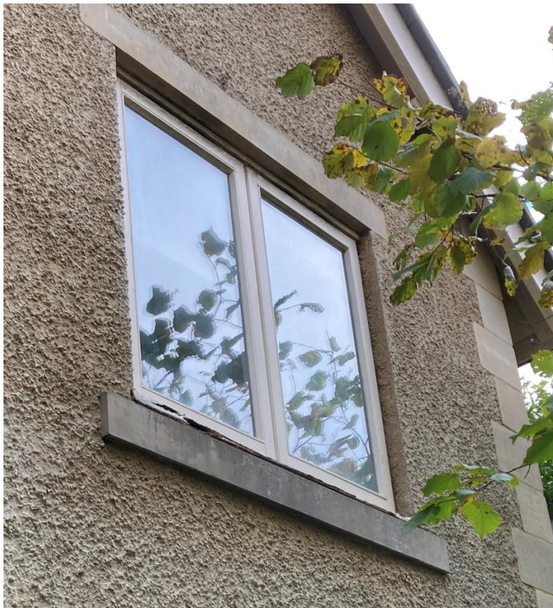
Figure 8: Window showing signs of deterioration, especially at cill
