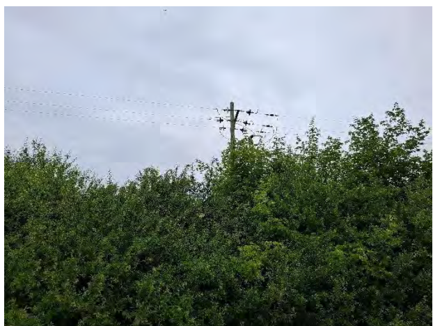
Photograph 18: Overhead service cables, northern boundary
