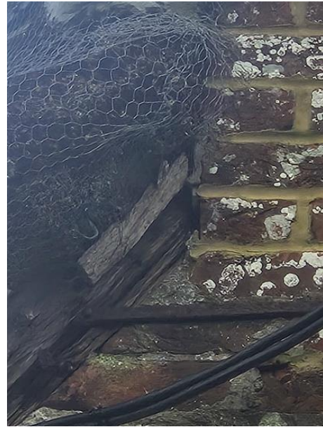
Photo 6: Gap on the western elevation of the cottage.
