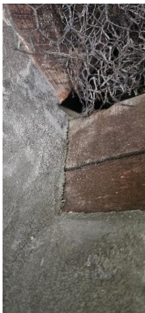
Photo 9: Small gap above fascia on southern elevation.
