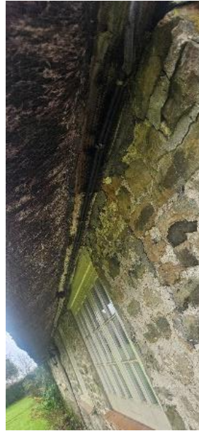
Photo 2: Closed eaves/fascia on northern elevation.
