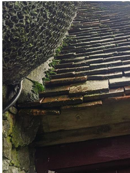
Photo 4: Gaps underneath tiles close to the cottage
