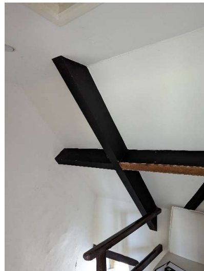
Figure 18: Photo of exposed purlin at first floor above staircase
