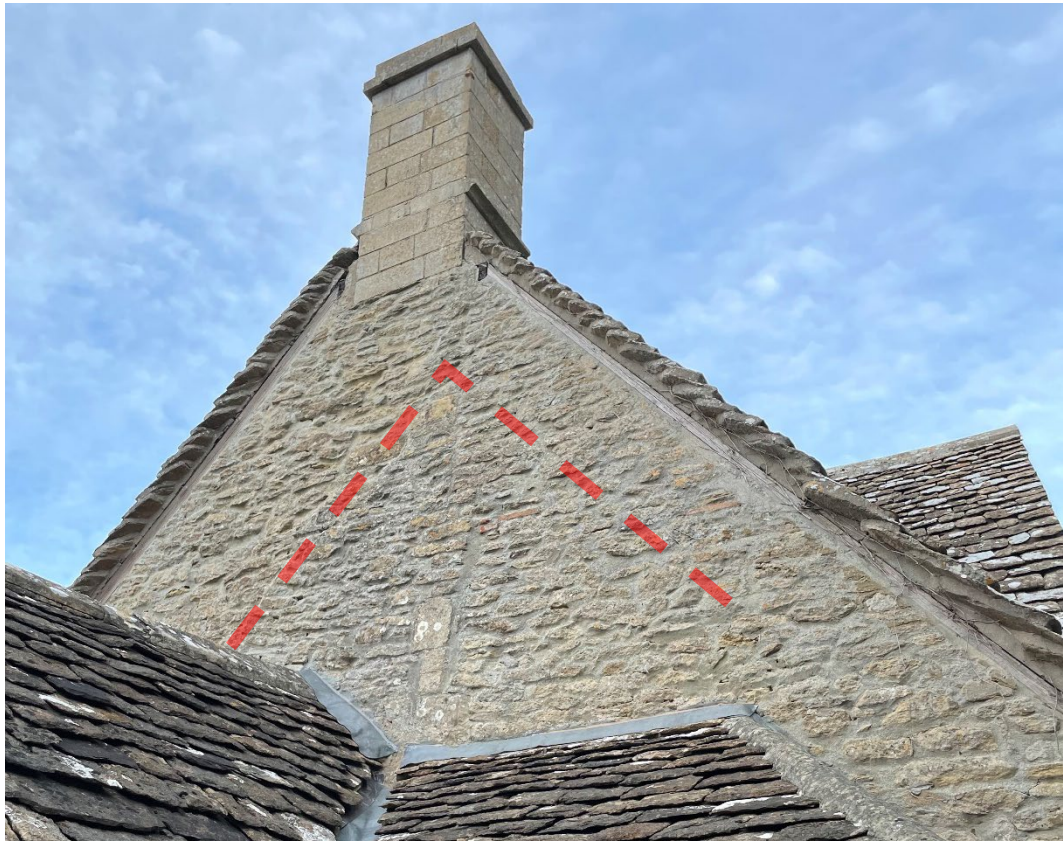
Figure 10: Western gable with slight straight joint highlighted where the stonework coursing changes slightly suggesting a former roof scar. Consistent later repointing somewhat obscures the contrasting build quality. Note rebuilt chimney.
