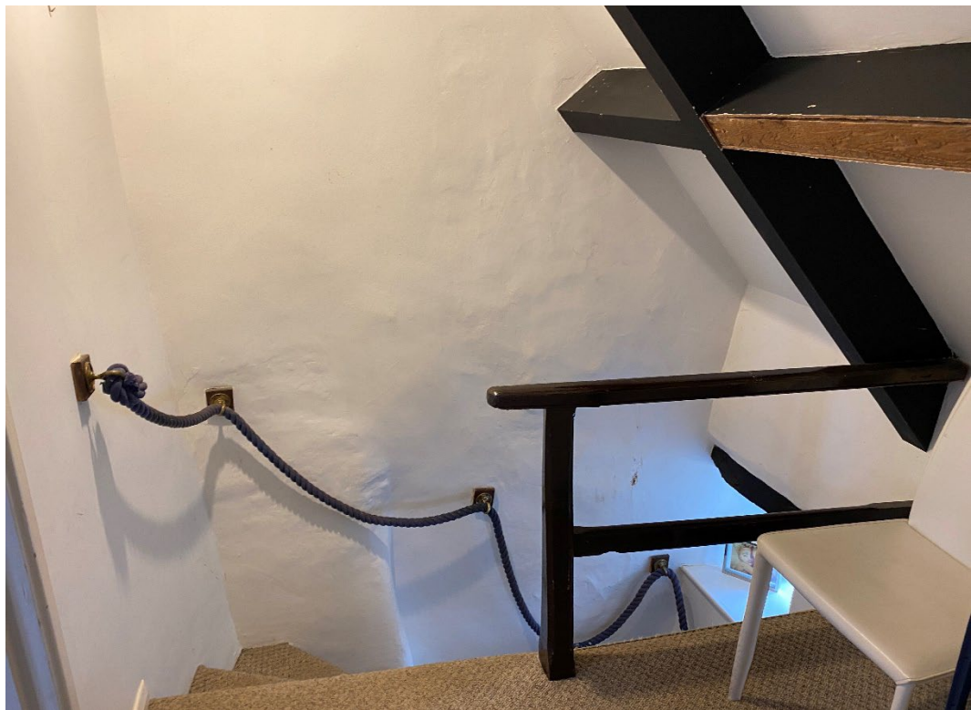
Figure 17: first floor landing at the head of the stairs with irregular plasterwork and, on the right, exposed replacement roof structure with plywood covering over soft wood timbers.
